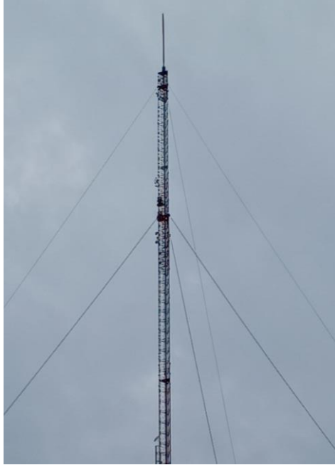
(a) Guyed tower
