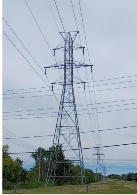
(b) power transmission networks
