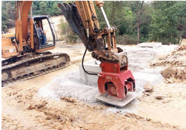
Figure 1.1. Backhoe Outfitted with Vibrating Plate Compacting Fill. Often this type of operation is performed hastily before an inspector can arrive at the site to check the quality of the compaction.
