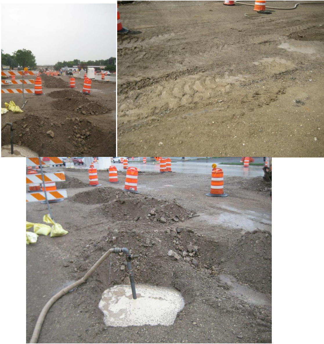
Figure 5.7. Pictures of Jetting Operation at Greenfield Avenue. Excavated Application Points (top left). Truck Compaction Treads After Filling Application Points (top right). Rigid Cast Iron Pipe Jetting Below Top of Subgrade (bottom).
