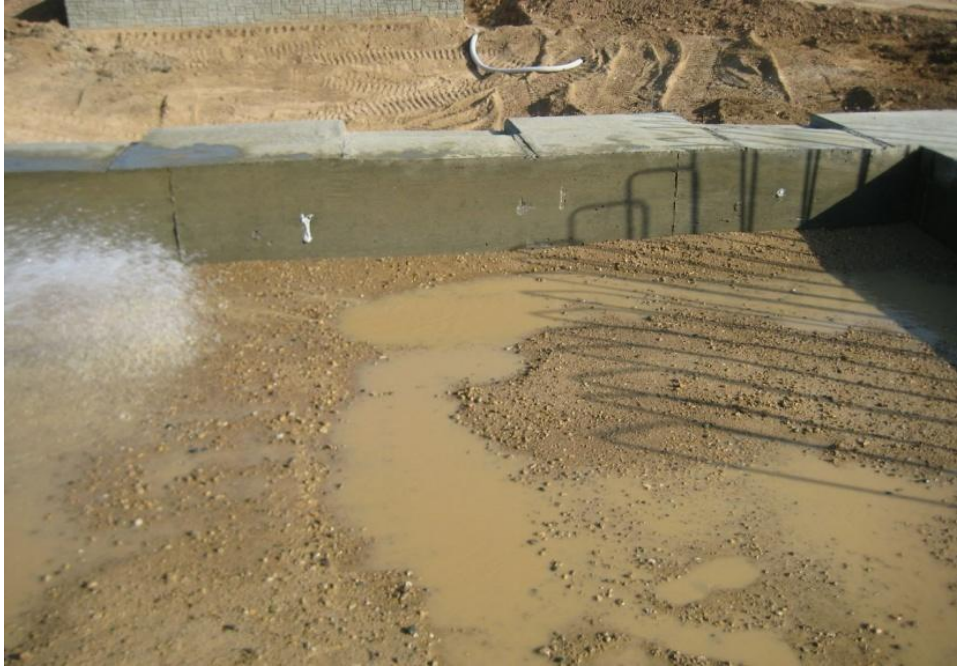
Figure 5.3. Ponding Observed on the Backfill Surface During Flooding. The picture here was taken 30 minutes after the water was turned on.
