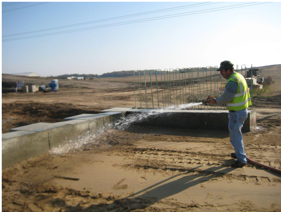
Figure 5.2. Flooding the Backfill to Initiate Compaction by Drainage. Just one water truck and one member from the contractor team was needed for the operation.
