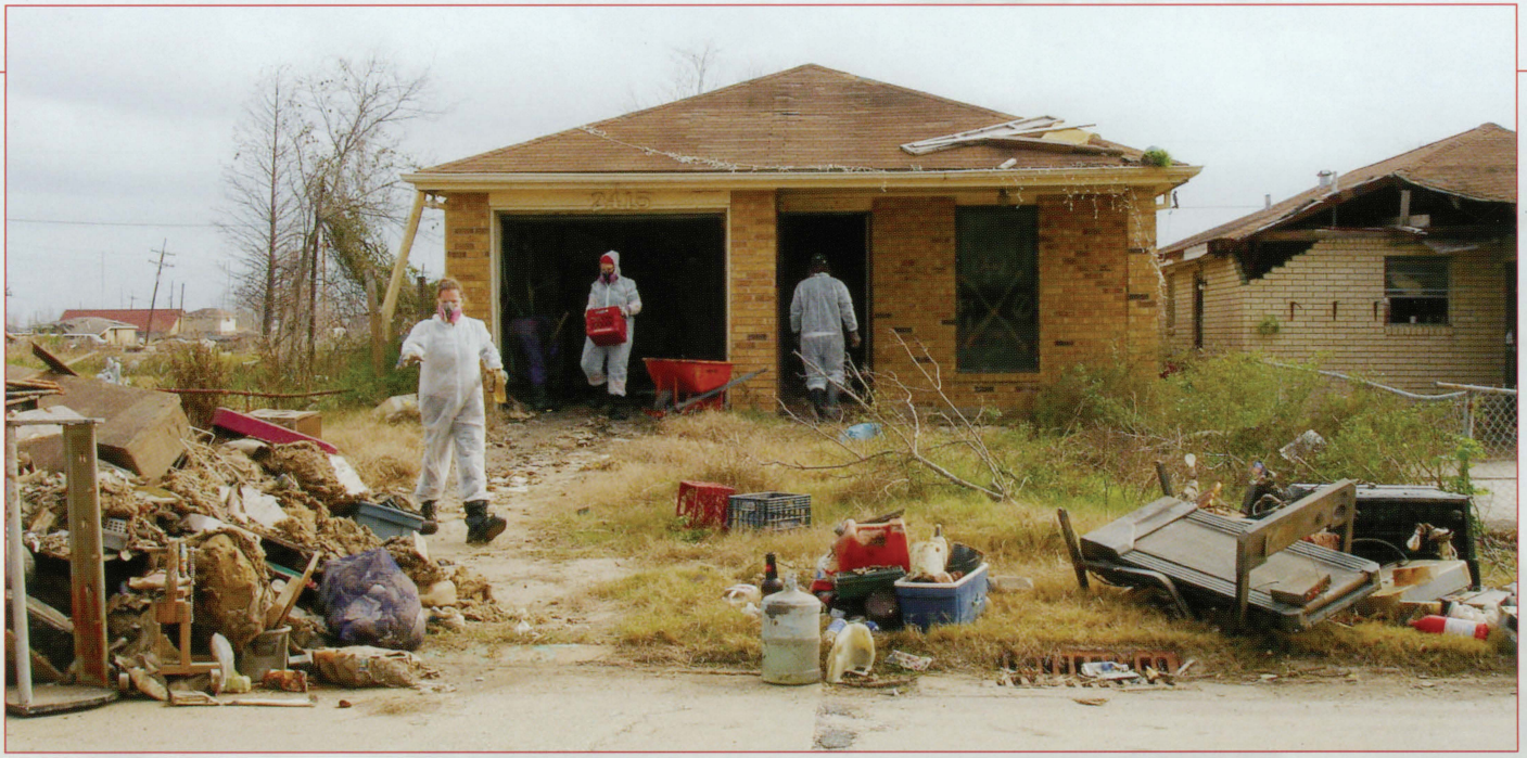
Gutting began with removing everything from each home—ruined items accumulated over time to maintain a household where a family once lived.
