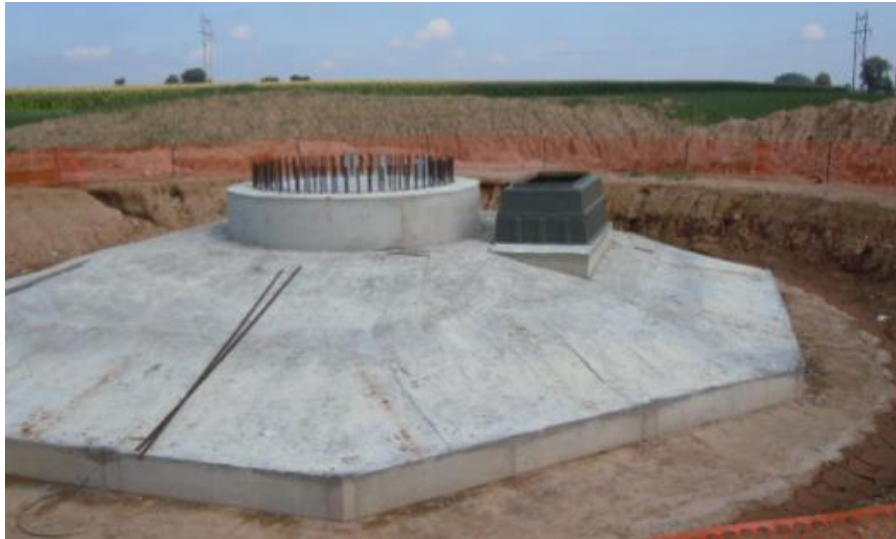
Figure 2-1: (a) Typical dimensions of a WTG shallow octagonal foundation and (b) construction of a shallow octagonal foundation.
