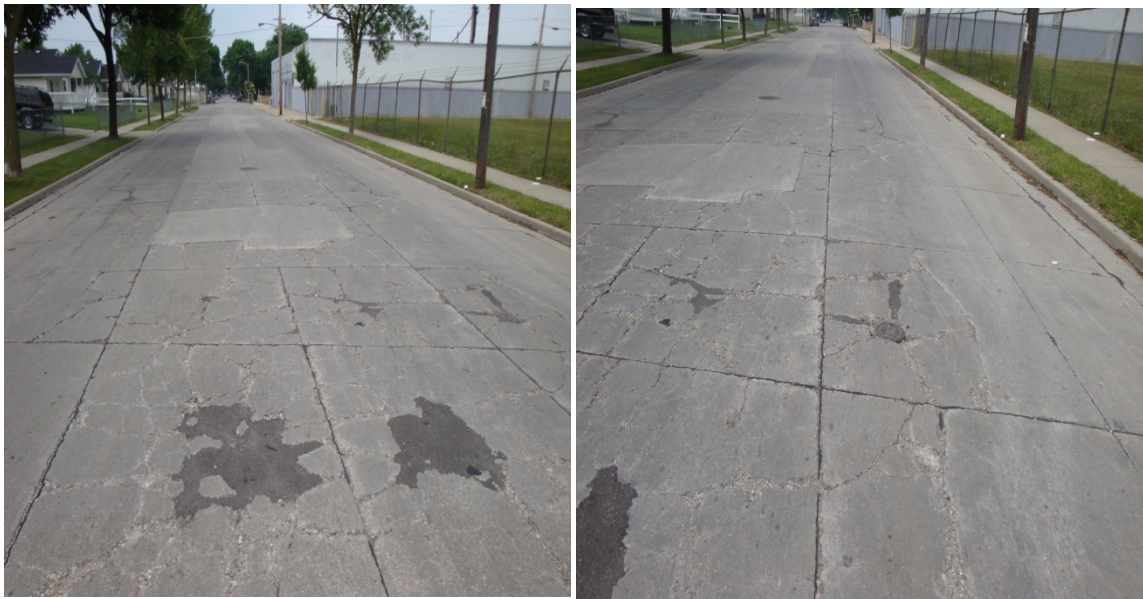
Figure 19. Condition of Galena Street (2009)
