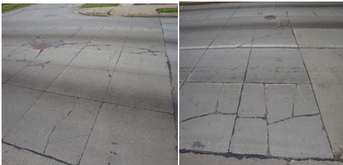
Figure 18. Condition of Fond Du Lac Avenue (2009)
