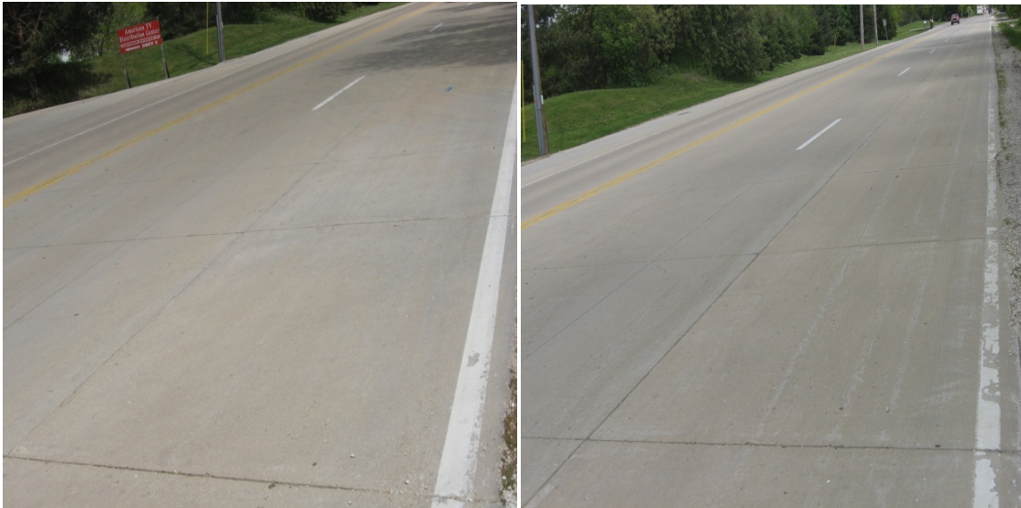
Figure 17. Condition of Duplainville Road (2008)
