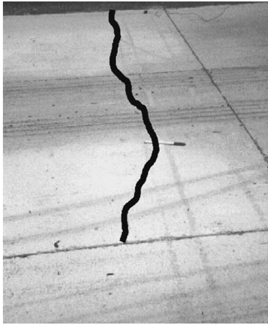
Figure 6. Mid-Slab Cracking (Rasmussen et al. 2002)
