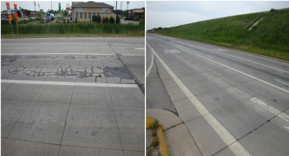
Figure 20. Condition of IH 94/STH 50 Ramp (2009)
