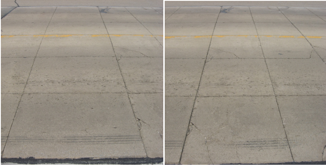
Figure 24. Condition of STH33 and CTH “A” (2008)
