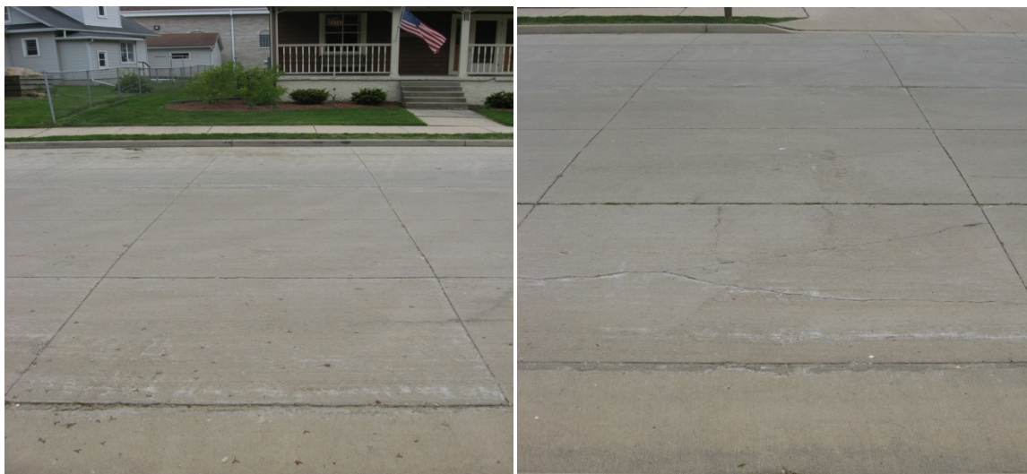
Figure 21. Condition of Lawndale Avenue (2008)
