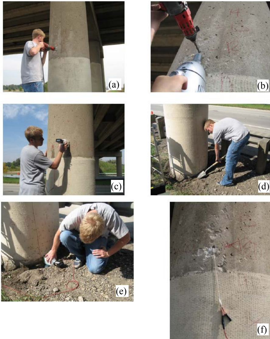
Figure 4.27: Half-cell potential and \text{Cl}^- content data and sample collection: (a) Concrete column drilling. (b) Concrete powder collection for \text{Cl}^- content estimation. (c) Half-cell potential measurements. (d) Access to the concrete column below the fiberglass wrap. (e) Half-cell potential measurements below the fiberglass wrap. (f) Electrode connection to steel rebar.
