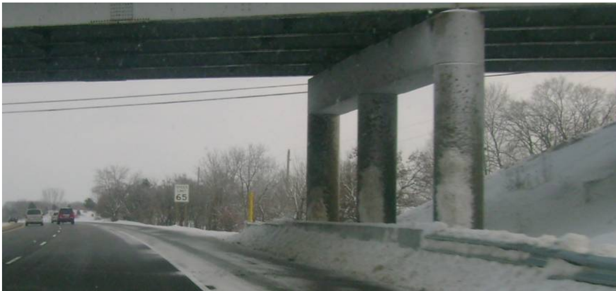
Figure 1.1: Snow and deicing solution splash on bridge columns (Interstate I-94 East bound – December 2008).
