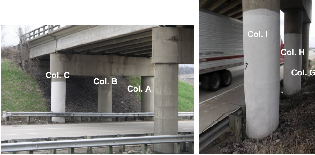
Figure 3.2: Location of B-11-17 bridge in Columbia Co., WI and arrangement of columns (map: after Google Maps 2008).
