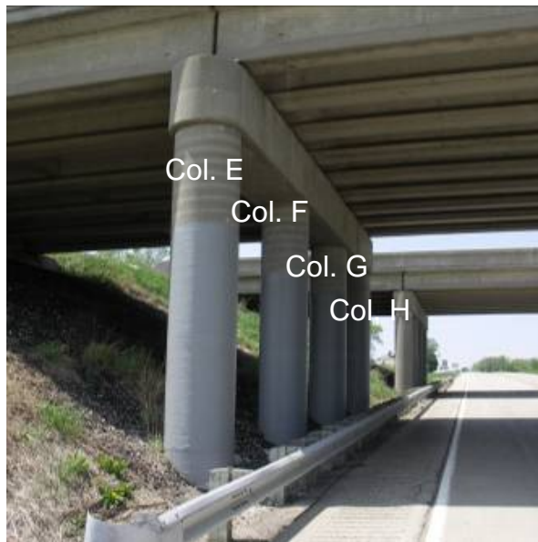
Figure 3.8: Location of B-11-172 bridge in Dane Co., WI and arrangement of columns (map: after Google Maps 2008).
