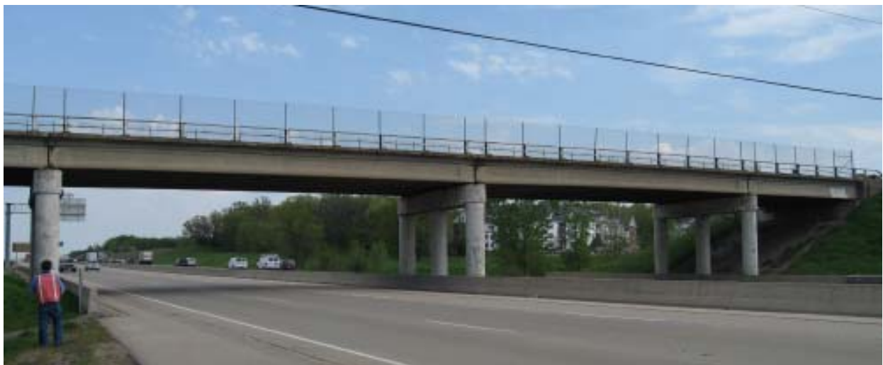
Figure 3.4: Location of B-11-113 bridge in Dane Co., WI and arrangement of columns (map: after Google Maps 2008).
