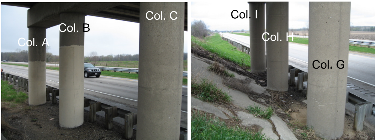
Figure 3.16: Location of B-28-45 bridge in Jefferson Co., WI and arrangement of columns (map: after Google Maps 2008).
