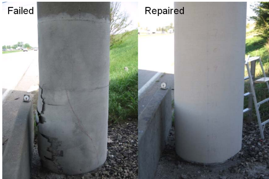
Figure 3.1: Evidence of corrosion activity in fiberglass wrapped column in bridge B-53-71 (I-39/90 under State highway 59). (a) May 2007 and (b) September 2007. After 10 years, WisDOT needed to re-wrap the column because corrosion continued under the fiberglass wrap.
