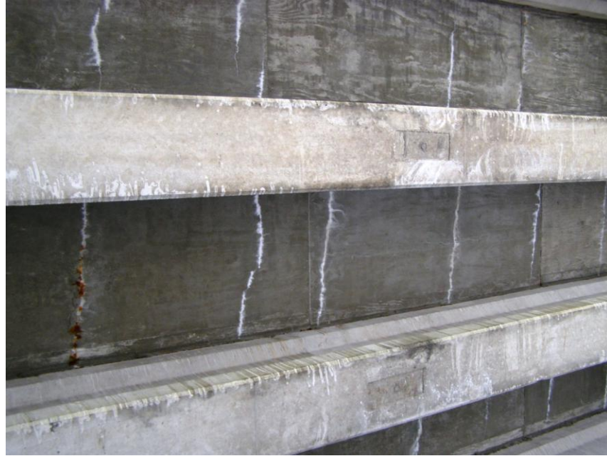
Figure 3.8 Evidence of efflorescence and rust stains on the underside of the deck of bridge B-13-0034.
