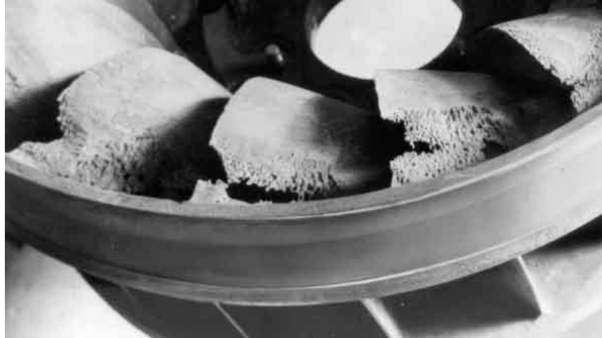
Figure 2: Cavitation damage on the blades at the discharge from a Francis turbine [9]
