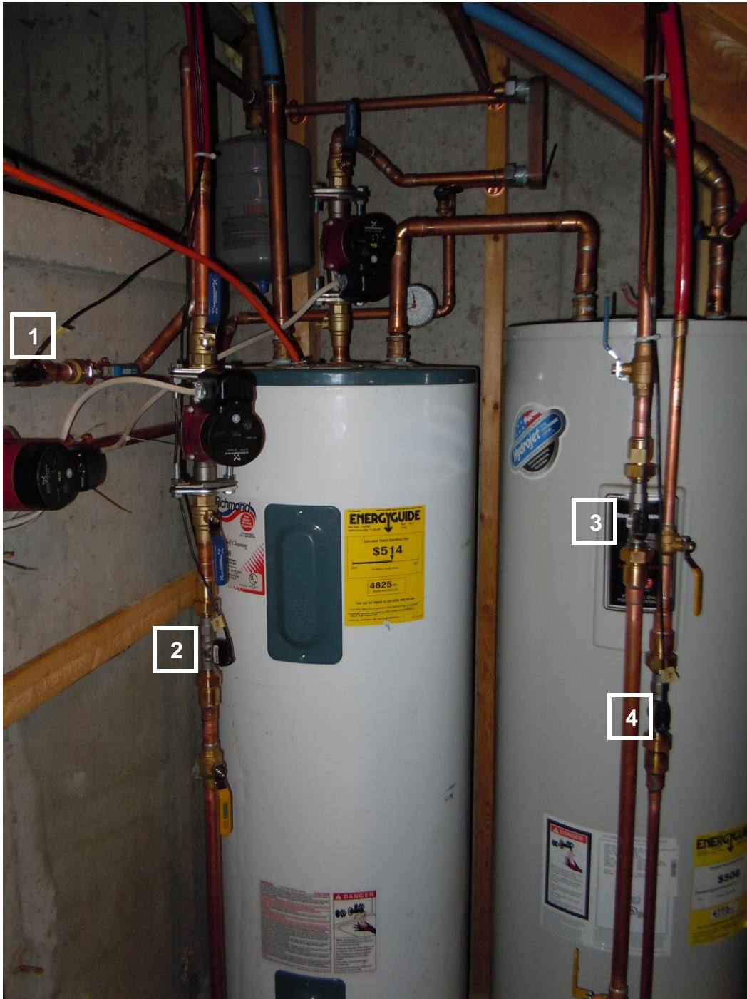
Fig. 10-5: Flow meter (1, 2, 3, and 4) placement near water storage tanks.
