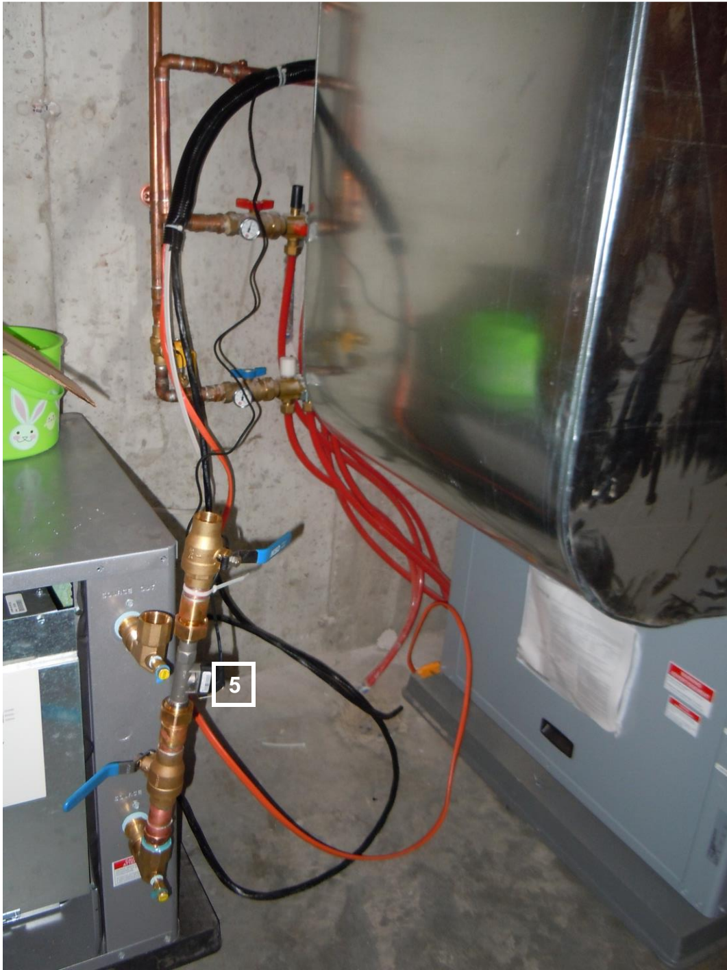
Fig. 10-6: Flow meter (5) placement near water-to-water heat exchanger.
