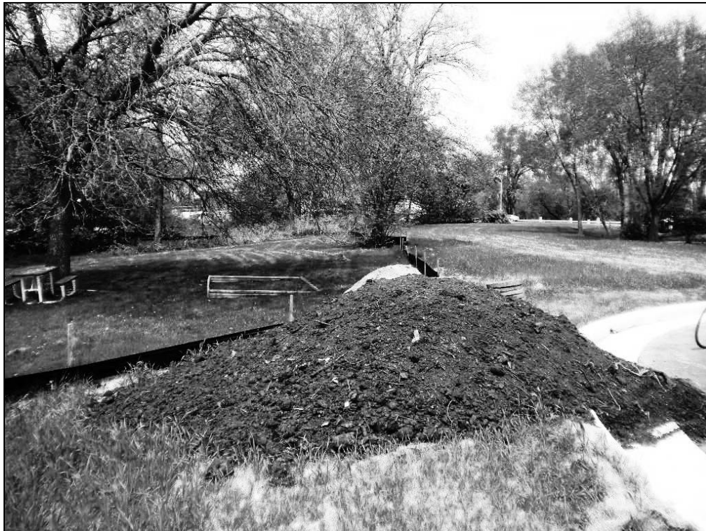
Photo 3 - McCormick Avenue filled with soil
