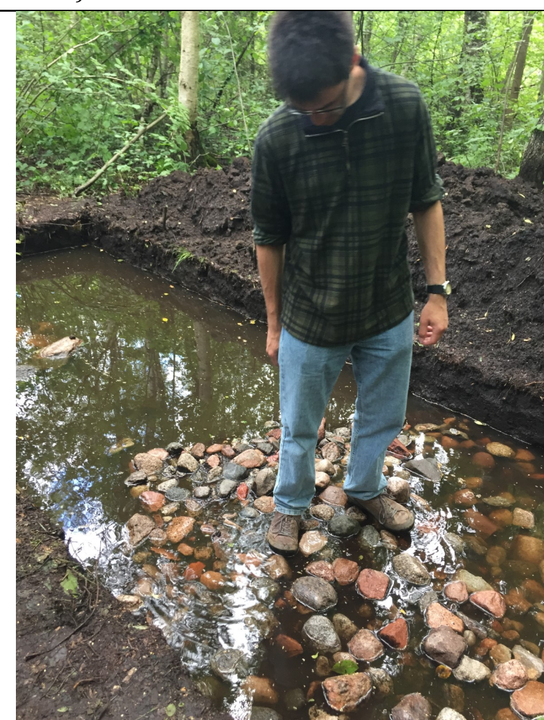
Excavation trenches quickly fill with water without specialized equipment which adds expense to a project. Knowing where to dig can save valuable time and money.
