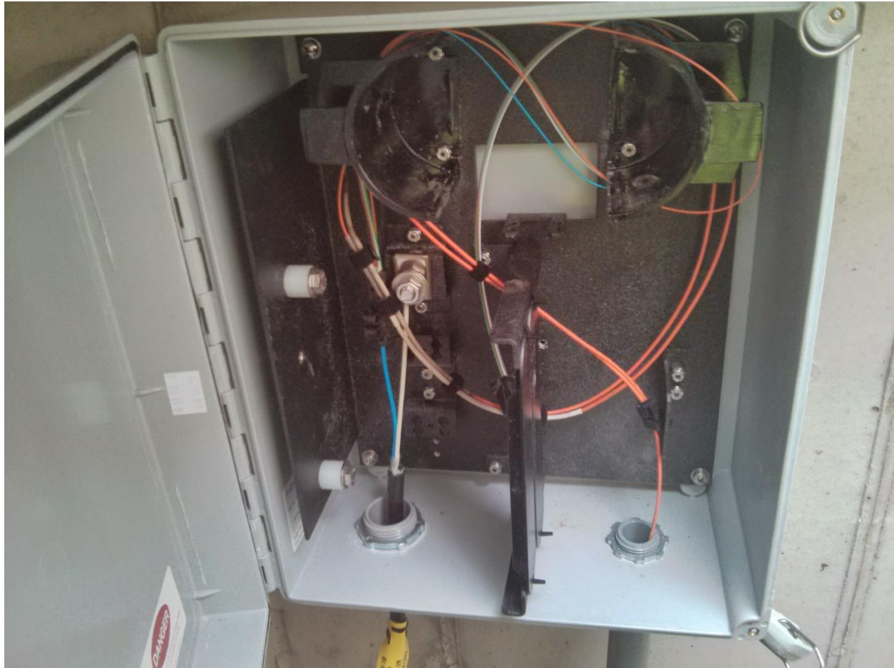
Figure 38: Photo of fusion splices as they appear in their enclosure at TMW-1B.
