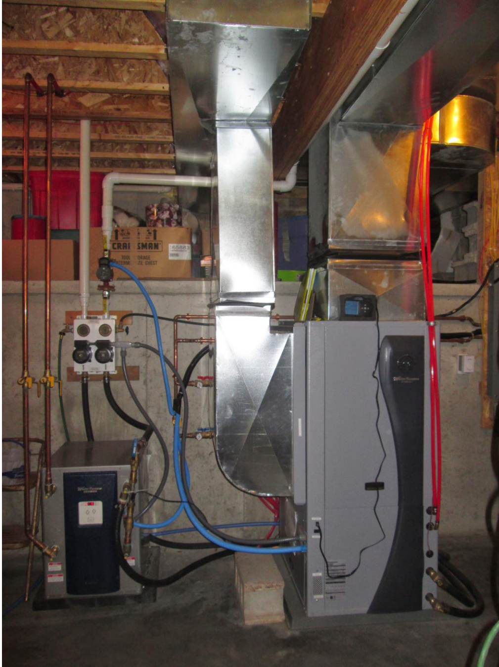
Figure 43: Photo of the two heat pumps at the site, water-to-water at left and water-to air at right. Copper pipes on left carry DHW to and from the water-to-water heat pump. The trio of circulation pumps at center circulate water to the water-to-water heat pump first before traveling to the water-to-air heat pump. Orange PEX tubing at right carry water to and from the desuperheater.
