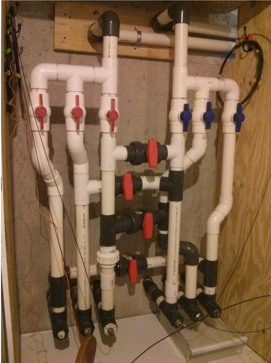
Figure 45: Photo of manifold. At bottom left, water returns to the three GHEs. At bottom right, water returns to the house. Water supply to and from the heat pumps is at top center.
