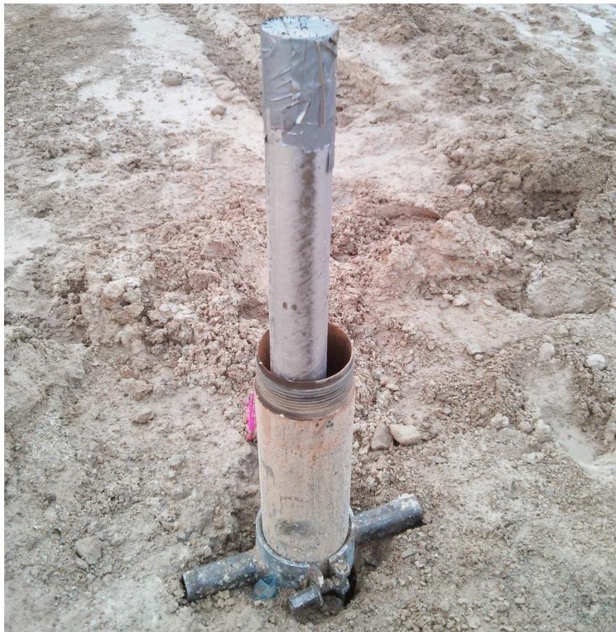
Figure 31: Fiberglass outer pipe of the coaxial GHE within the borehole casing before inner tubing was installed.
