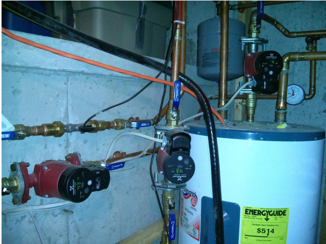
Figure 44: DHW storage tank and associated circulation pumps. At left, pump circulates water from plate heat exchanger to underfloor heating. At center, pump circulates water from DHW tank to water-to-water heat pump. At right, pump circulates DHW to plate heat exchanger.
