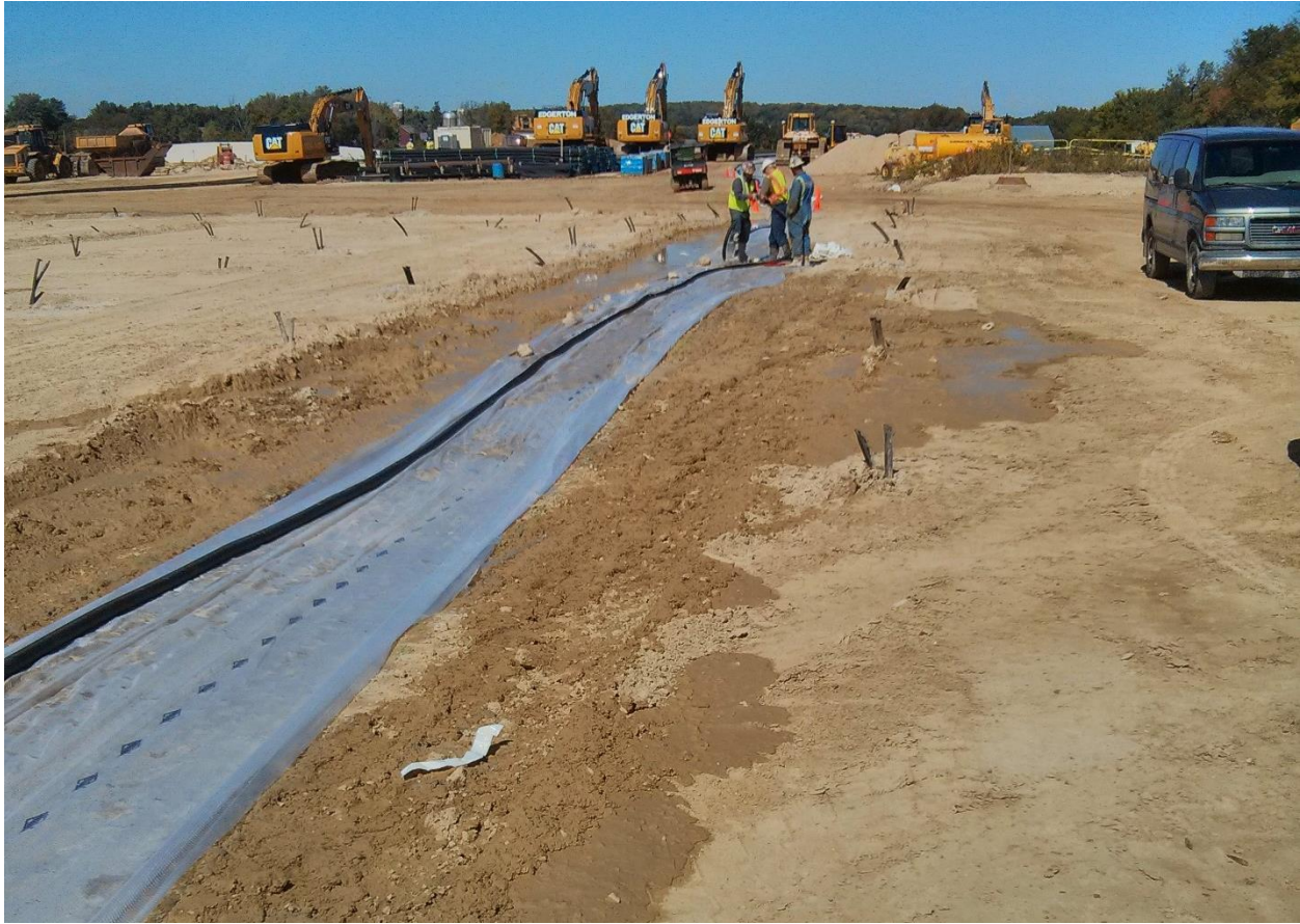
Figure 32: Laying out sections of the inner tube for the coaxial GHE before fiber was strung through the inside and wrapped on the outside.
