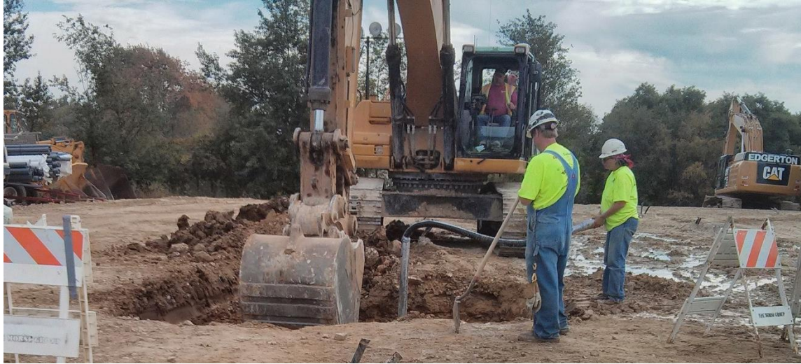
Figure 34: Excavating around the GHE to make room for the vault and well-head (~2 m depth).
