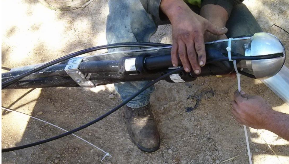
Figure 29: Torpedo being prepared for the installation of the instrumented u-tube heat exchange well. This photo is also representative of the torpedoes used on the sentry well fibers, though those obviously did not include heat exchange pipe as in this photo.
