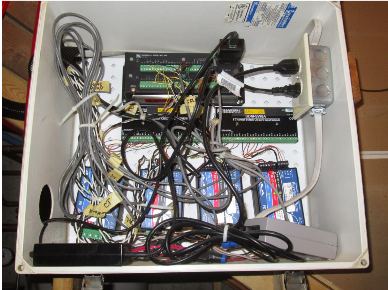
Figure 42: Photo of CR10X datalogger (top), switch closure modules (middle), and WattNodes (bottom) after connecting flow meters (black) but before connection of all system monitoring equipment.
