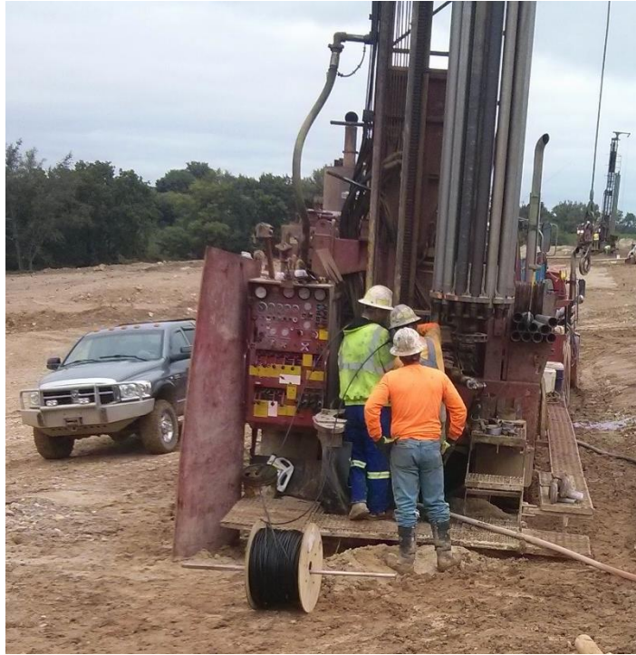
Figure 30: Coiled fiber protected in HDPE tubing is affixed to rig weight bar before being dropped to the bottom of sentry well TMW-2B.
