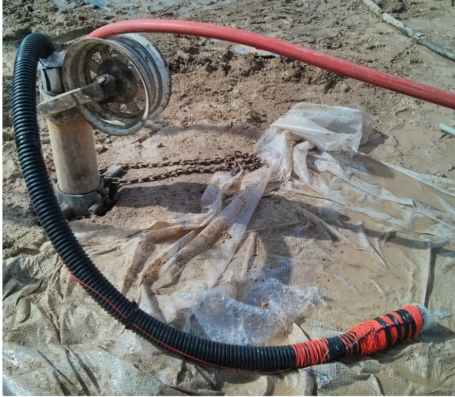
Figure 33: Inner tube of the coaxial system placed within the fiberglass outer pipe while the outer pipe is grouted within the borehole (tremie pipe in red). Fiber travels down the inside of the tube and back up the outside. Excess fiber (orange) was wrapped on the end of the tube and later covered to protect it from the rough edges of the steel casing as it was pulled.
