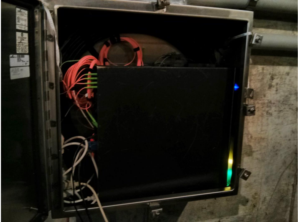
Figure 26: Halo DTS interrogator as installed in a NEMA enclosure in Vault 14 on December 3, 2014. Four E-2000 APC connectors are connected at the top left of the interrogator.
