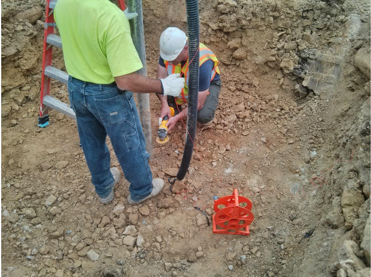
Figure 35: Careful trimming of the pipes for the GHE. Special care had to be taken to only cut the pipes and not the fibers. After the pipes were cut in a horizontal plane, they were cut in the vertical plane so that the excess fiber could be pulled out.
