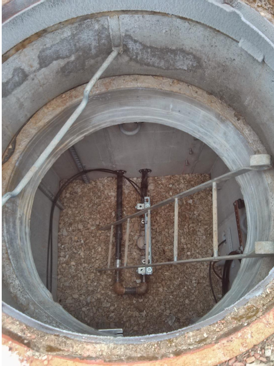
Figure 39: An example photo of the wellhead vaults employed at Borefield #4. This photo was taken at the coaxial GHE wellhead. The black pipe carries supply and return water to and from the coaxial GHE. The black tubing carries the fiber out of the GHE to the fusion splice panels. The opening is a standard manhole (~1 m). The floor is slightly larger at 1.2 m x 1.2 m.
