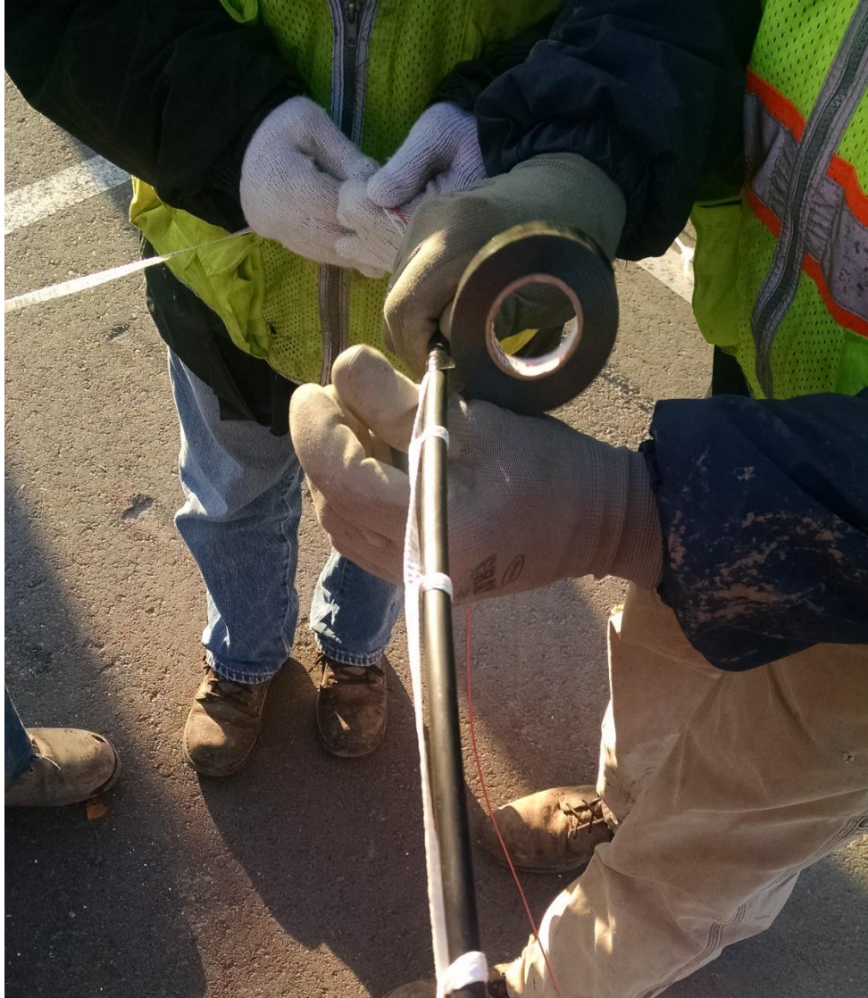
Figure 37: Pull string being taped to the fiber's protective tubing. The excess calibration fiber was allowed to trail behind the pull string as the tubing was pulled through.
