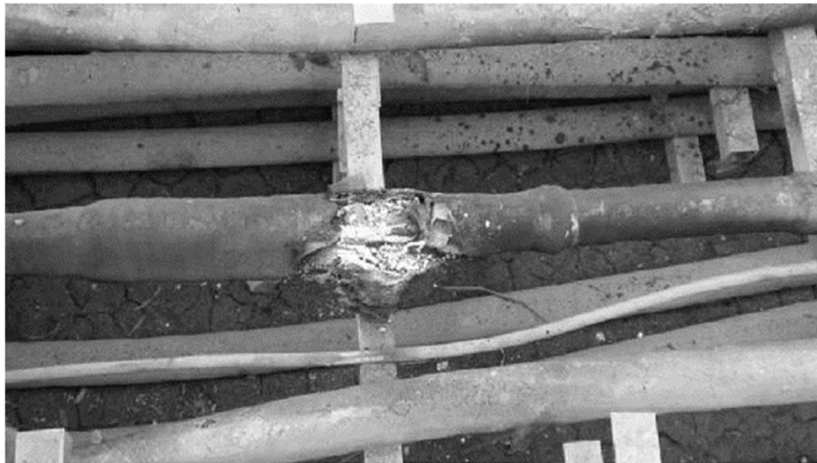
Figure 1-2 Corrupt Cable that Cause Ground Fault
