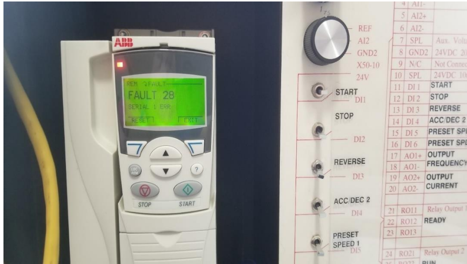
Figure 5-19. ABB drive error with “FAULT 28”
