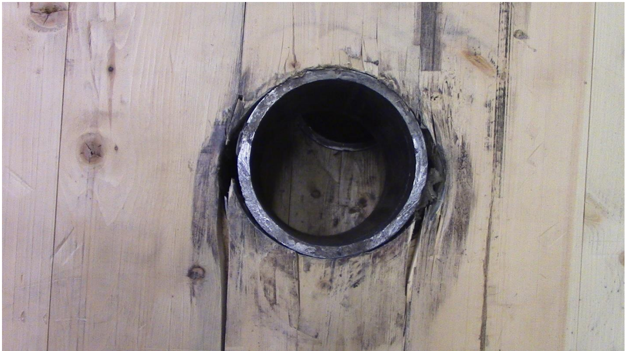
Figure 85. Damage and elongation of hole around pipe bushing of ( e = 0.94 ) panel.
