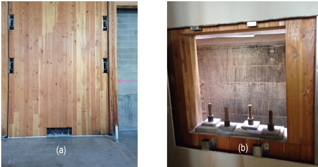
Figure 11. Vertically post-tensioned (PT) CLT wall with UFPs Viewed at (a) ground floor and (b) top of wall PT anchorage. Peavy Hall, Oregon State University
