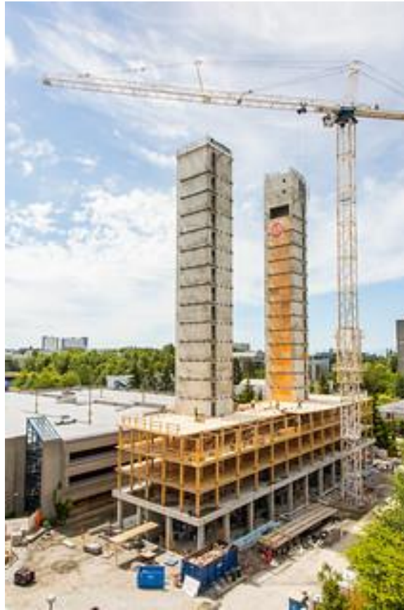
Figure 4. Construction of Brock Commons pairing timber with reinforced concrete Source: (Aston Ostry, UBC Media Relations)
