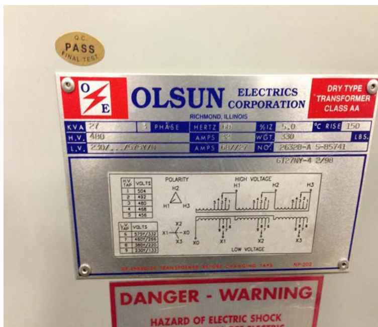
Figure 4.2: Power Transformer Data Nameplate
