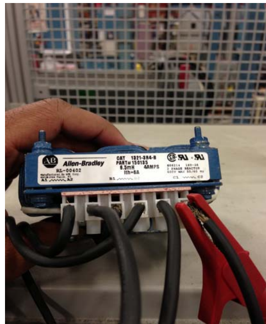
Figure 4.10: Line Reactor Used to Create Voltage Unbalance
