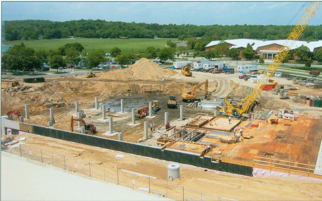
The Health Sciences Learning Center continues to take shape immediately adjacent to UW Hospital and Clinics, with work proceeding on the building's foundation system. At left, the foundation for the lower-level garage is being completed, while on the right of the photograph the formwork for the ceiling of the garage is being finished. Both areas comprise what will be the Education Wing. Just north of this area, excavation for the lower level of the Library Wing is beginning.
