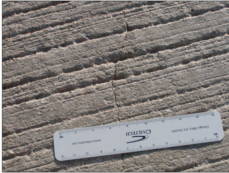
Figure 3.21 (6) Hairline Crack on Deck of B-20-149 with Scale
