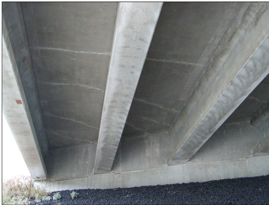
Figure 3.16 (24) Underside of Bridge Deck at North Abutment, Girders (From Left to Right) 1, 2, and 3, B-20-134
