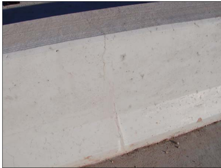
Figure 3.34 (5) Northern Parapet Crack on B-20-149
