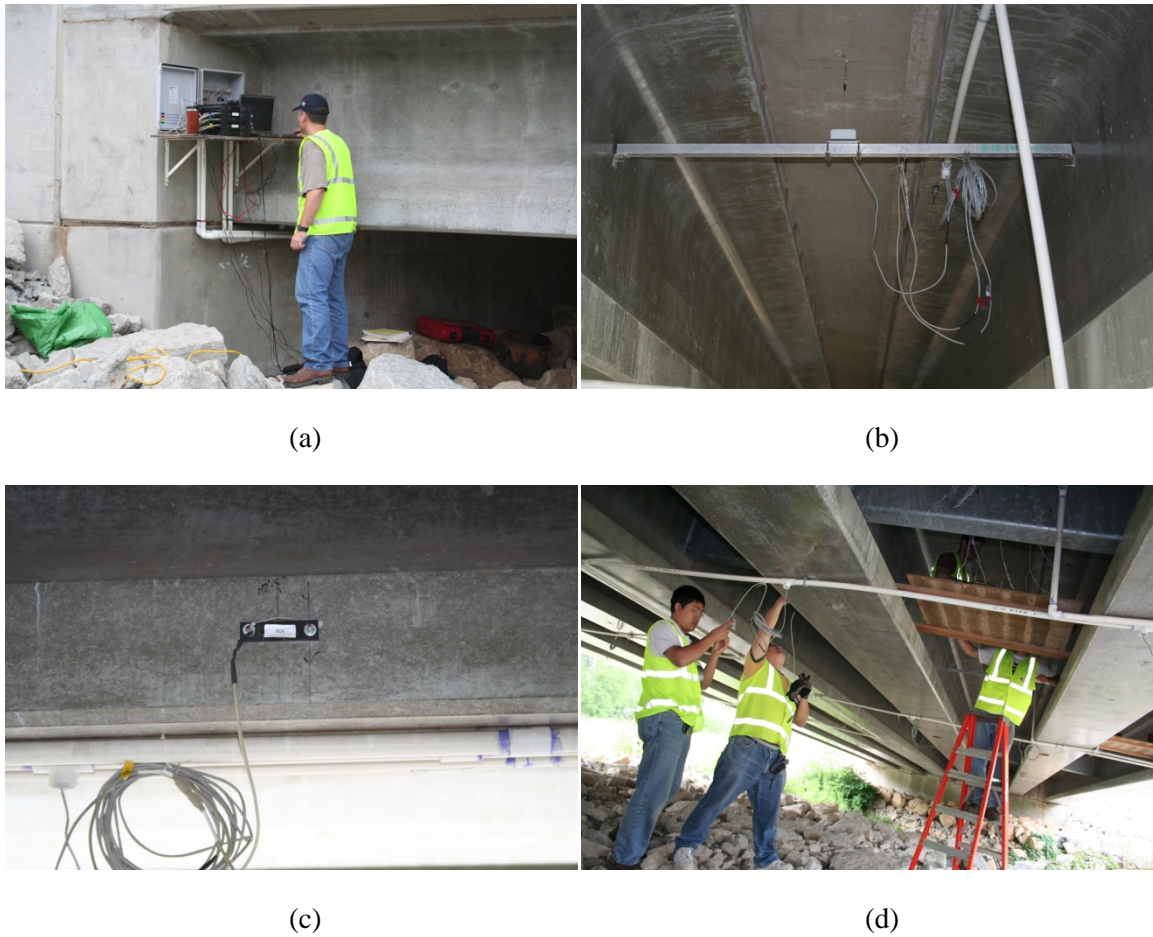
Figure 4.12 B-20-148 Data Acquisition System and Instrumentation: (a) Data Acquisition System and Enclosure; (b) Draw Wire Transducer Installation; (c) Strain Gauge Installation; (d) Sensor Wiring Runs and Sensor Installation.
