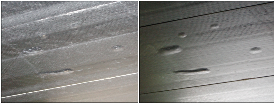
Figure 3.15 (9) West Span Blisters and Sealant Seep-Through in FRP-SIP Deck Between Girder 3 and 4 Near West Abutment, B-20-133
