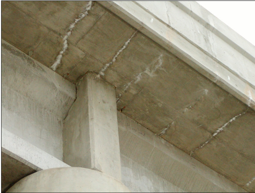
Figure 3.7 (3) Cracking with Efflorescence South Side of B-20-133 Above Central Pier
