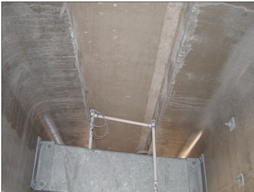
Figure 3.33 (19) First Diaphragm under B-20-148 Between Girders 5 and 6 with Wiring for Load Testing
