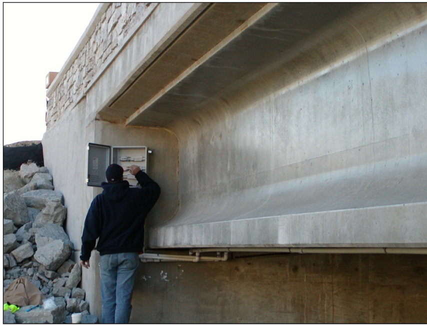
Figure 3.26 (16) East Abutment on North Side of B-20-148 with Data Acquisition Box Looking SW
