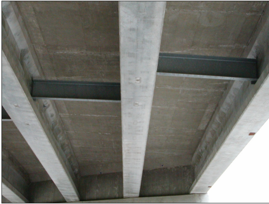
Figure 3.17 (26) West Span Looking East at 1 st diaphragm, Girders (From Left to Right), 3, 2, and 1, B-20-134
