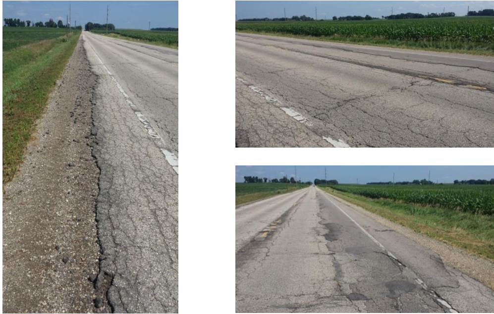
(b) Pictures of various pavement surface distresses
