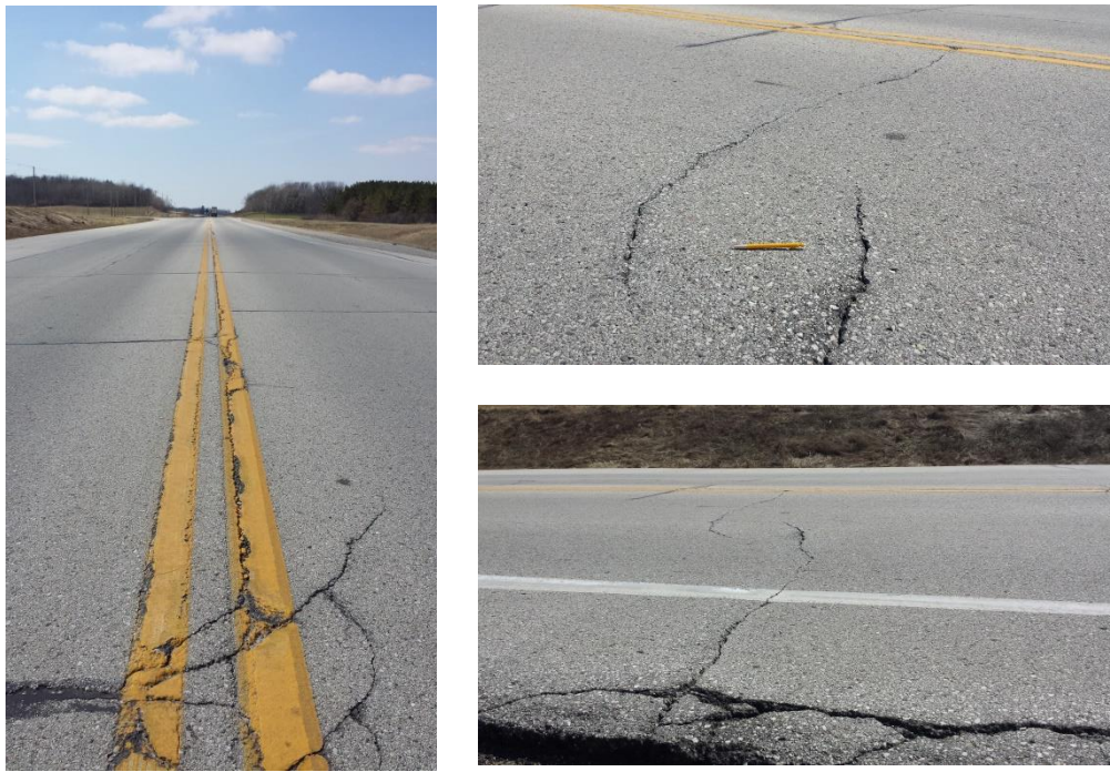
Figure 4.16: Pavement surface distresses observed on STH 23
