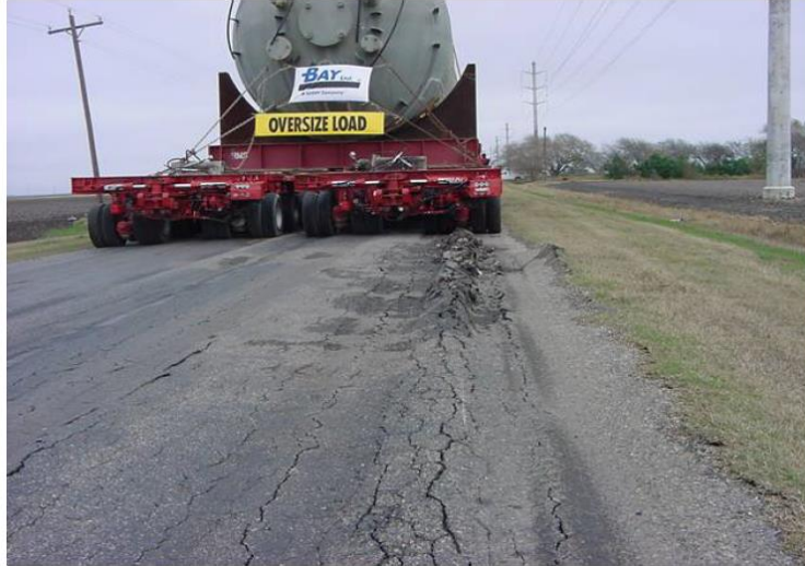
Figure 2.3: Pavement Damage to Farm to Market Road 796 in Texas (Oh and Wimsatt 2010)
