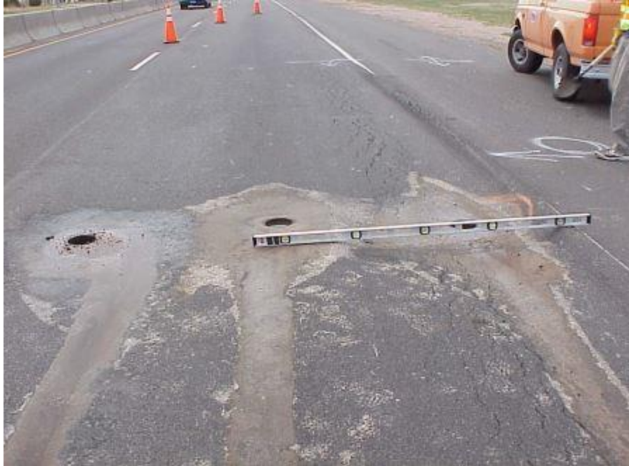
Figure 2.8: Rutting along Vazquez Boulevard in Commerce City, CO (Acimovic et al. 2007)
