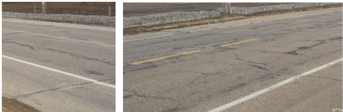
Figure 4.14: Pavement surface distresses observed on STH 11
