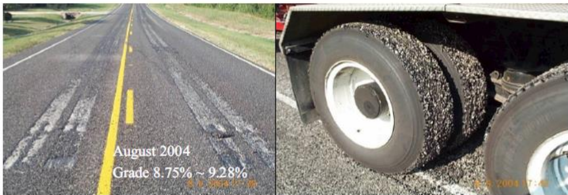
Figure 2.6: Pavement Damage on Farm to Market Road 109 in Texas (Chen et al. 2009)
