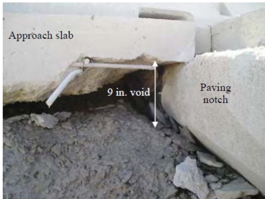
Figure 2.6 – Settlement trench observed from rehabilitation project (White et al. 2005)
