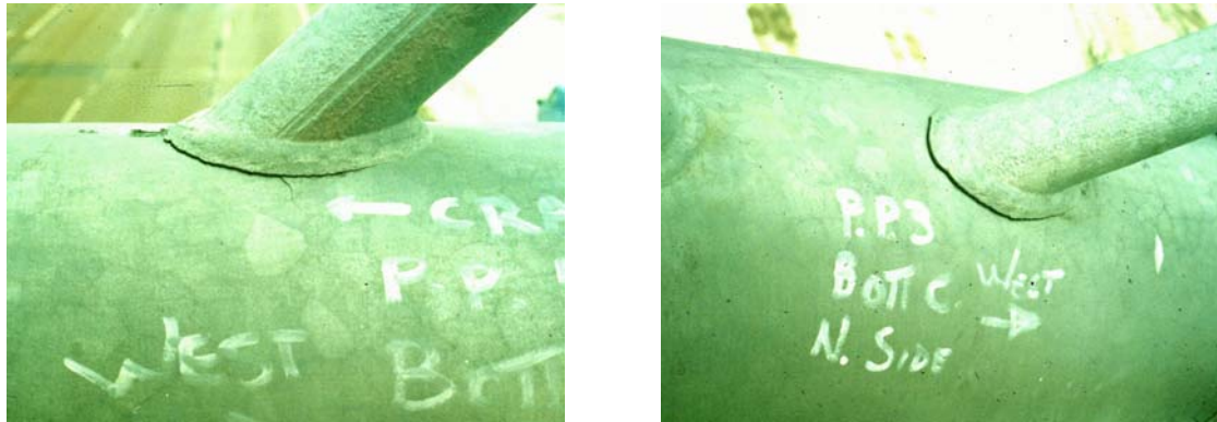
Figure 2.30: Typical Cracking Observed During Sign Support Structure Service Life.
