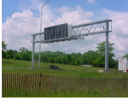
Figure 3.5: “Minnesota Design” currently used by WisDOT to Support VMS.
