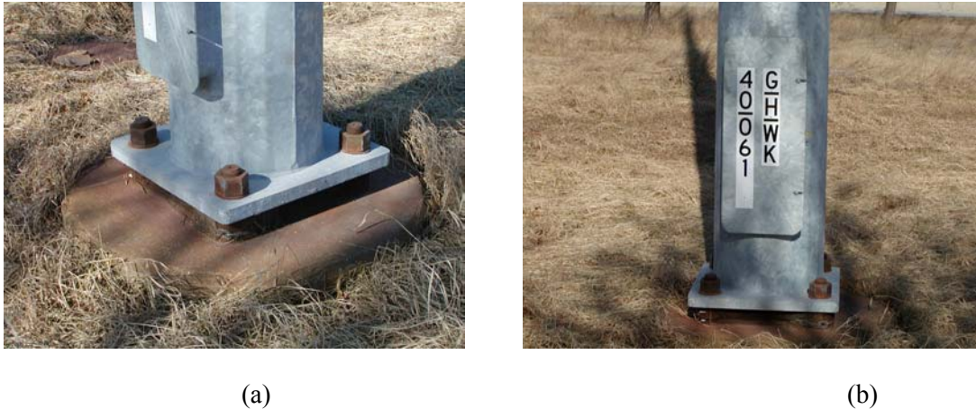
Figure 3.44: Base Plate Arrangement for HML-40-061: (a) Existing Anchor Rods and Pattern; (b) Hand-Hole and Mounting Plate.
