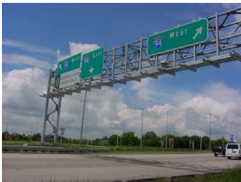
Figure 3.4: Four-Chord Bolted Angles and Welded Gusset Plates Truss Configuration currently used by WisDOT.
