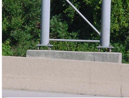
Figure 3.16: In-Service Base Plate Condition of Sign Bridge S-67-402 (Ginal 2003).
