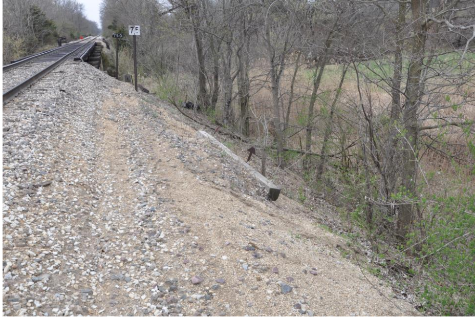
Figure 28: Mile Marker 75. Note: Ballast and shoulder washout with support structure
