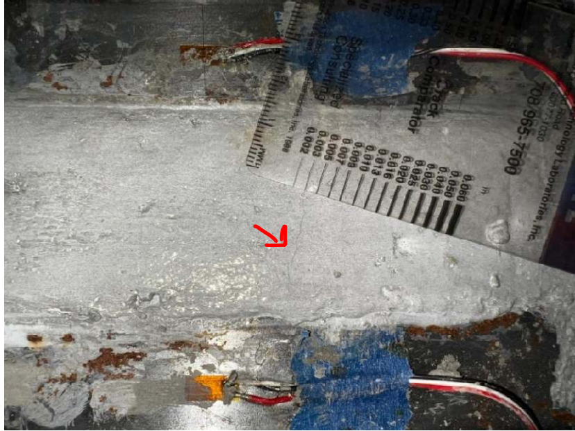
Figure 28 Crack formation on the 3-day wet-cured specimen
