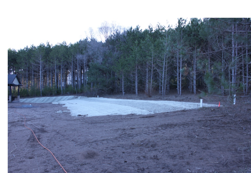
Fig 6. Typical Huntsinger Heights septic system absorption field. This newly constructed absorption field is located in the glacial outwash on the south side of lot 19 (Fig. 7)
