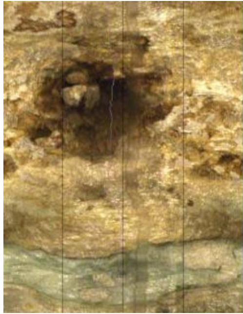
Figure 17: 360 degree view of the 0.4 m void just below the water table at 30 m bgs.
