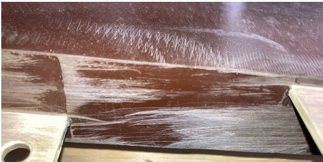
Figure 3.10: Surface Roughness of the Laminated Bus Bar
