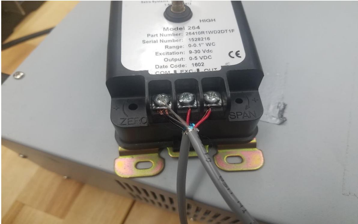
Figure 7.20 Pressure transducer connection.
