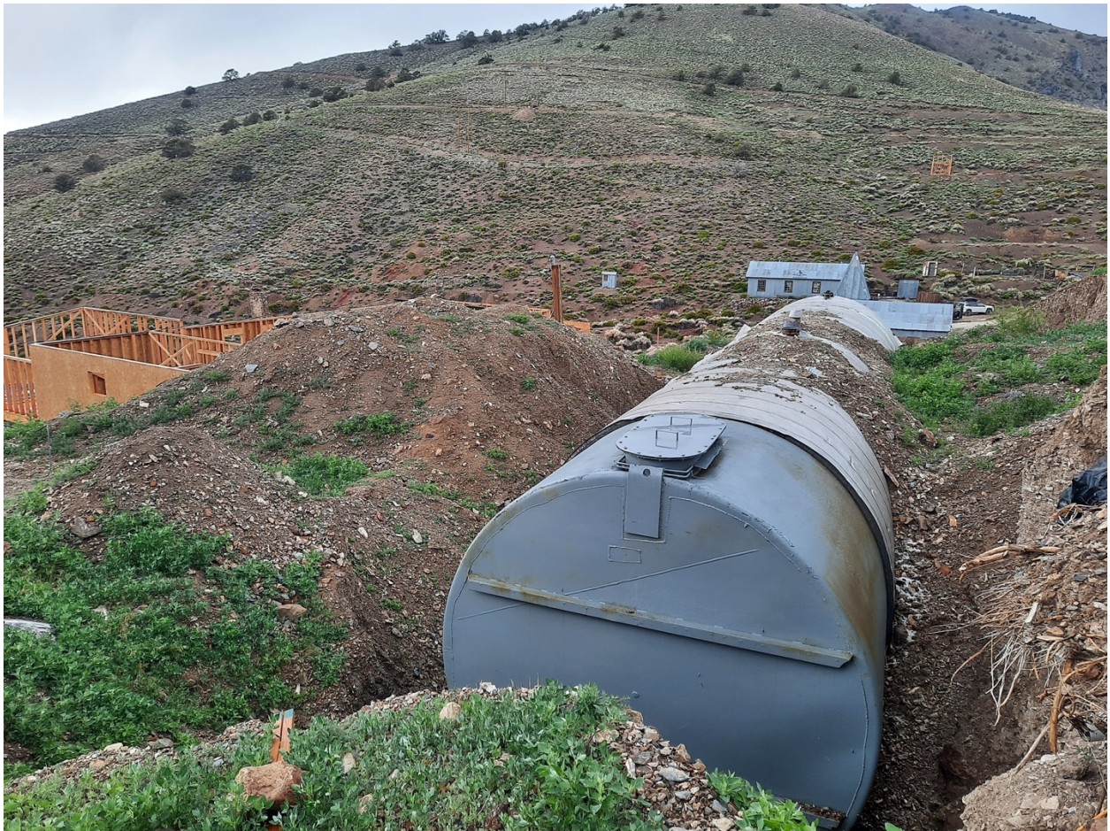
Figure 33: 40,000 gallon water tank.
