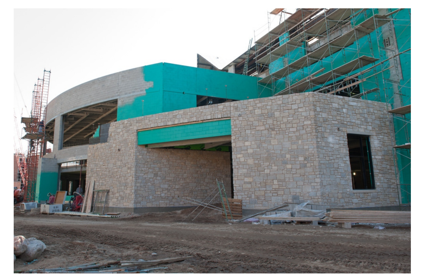
Dolomite dimension stone being applied to the exterior of W.R. Davies Student Center during construction in the Spring of 2012.
