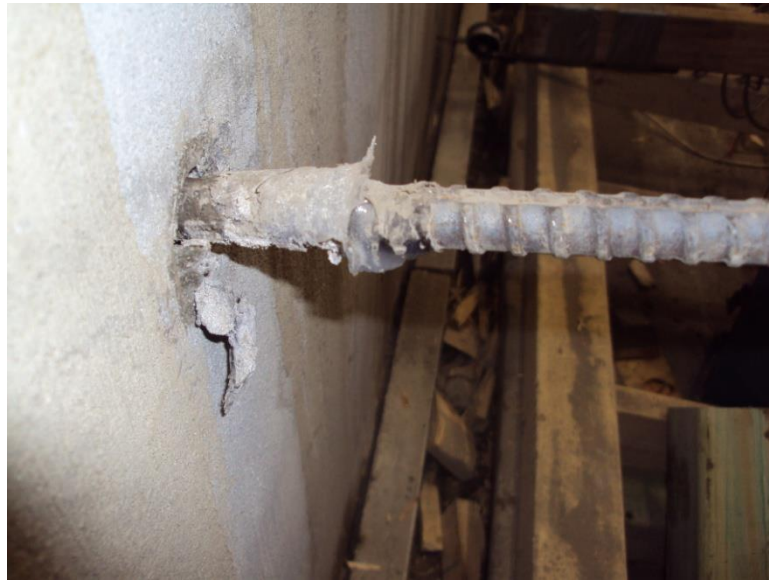
Figure 3.34: Pullout failure of rebar in CLSM abutment.
