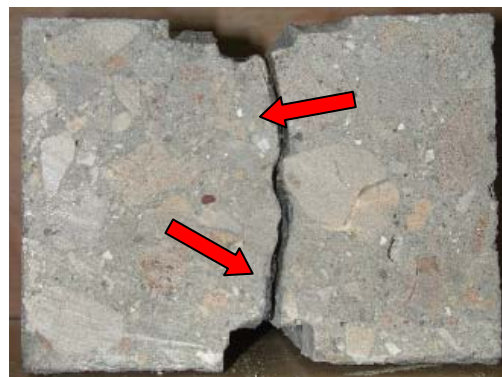
Figure 4.2.4 Example of a sealant failure.
