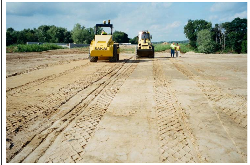
Figure 31. Jefferson STH 18 Project; Bomag and Sakai IC Rollers Used to Compact the Low Plasticity Clay and Silty Sand Embankment
