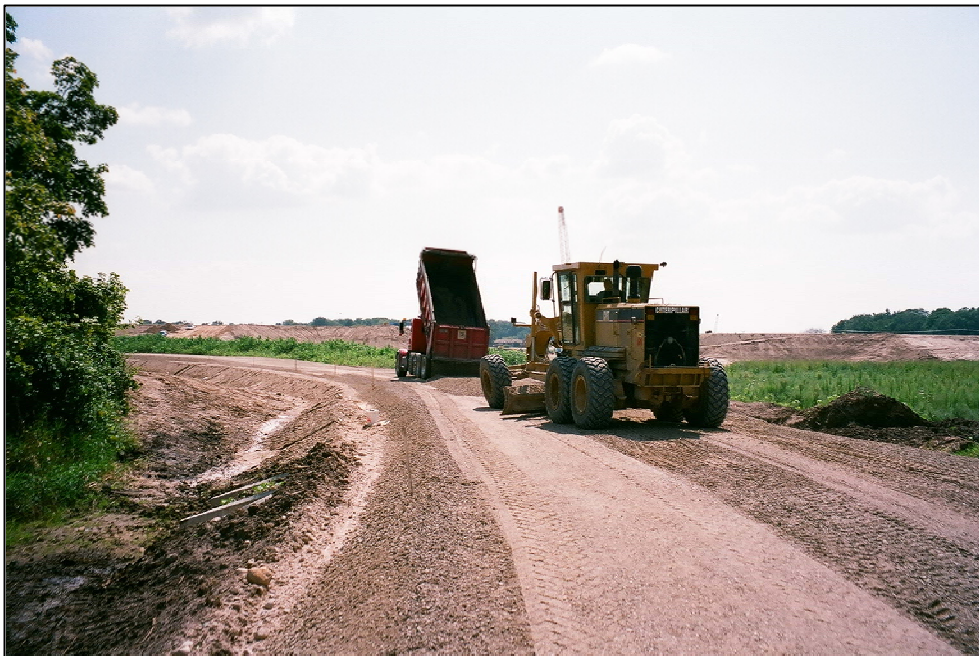
Figure 32. Jefferson STH 18 Project; Placement and Spreading of the Second Lift of Crushed Aggregate Base (Both Lifts Were Included in Project)
