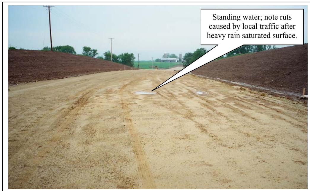
Figure 22. Highland STH 80 Project; Granular Embankment Test Section, Saturated with Standing Water from Heavy Rains and Excluded from Demonstration Project
