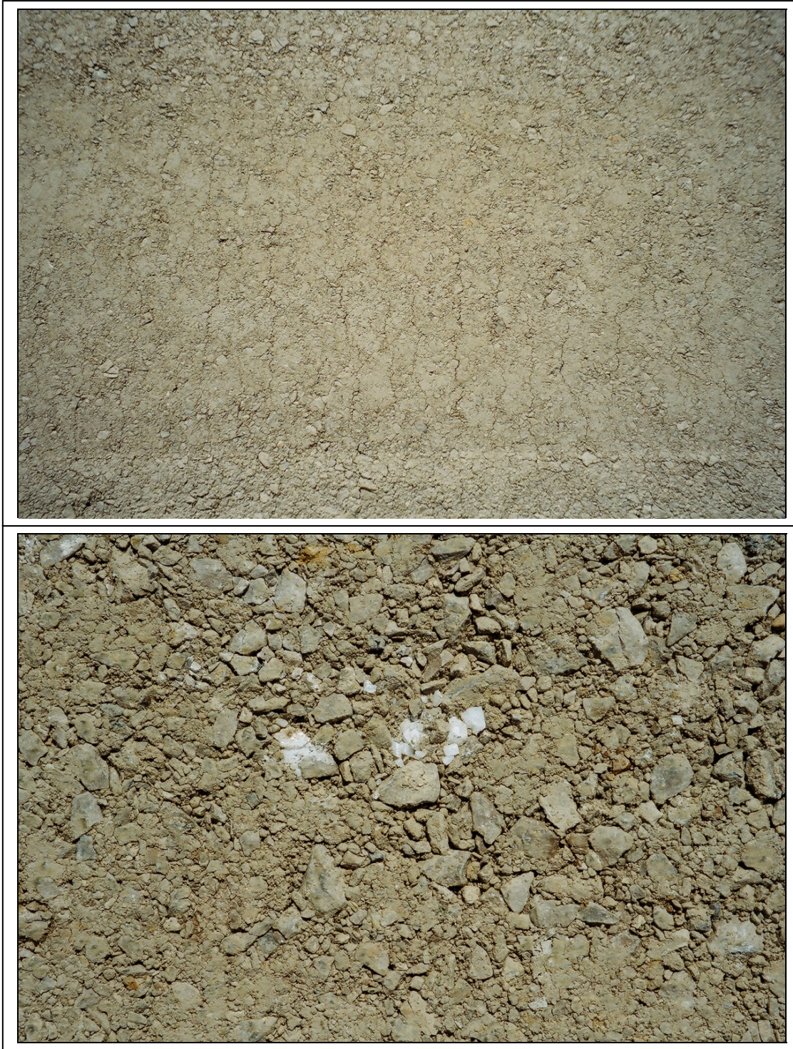
Figure 69. Jefferson Project; Photographs of the Crushed Aggregate Base Surface Showing the Cracks and Crushed Aggregate
