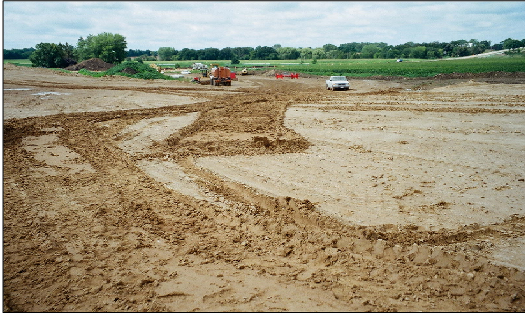
Figure 28. Jefferson STH 18 Project; Embankment Test Area After Heavy Rains
