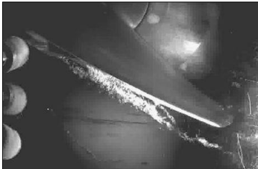
Figure 10: Severe cavitation erosion as witnessed on a Francis turbine [22]
