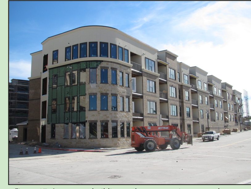
Figure 17. Apartment building under construction across the street from Dr. Pepper Ballpark (2003) in Frisco. Photo: Ezra Zeitler, 2013
