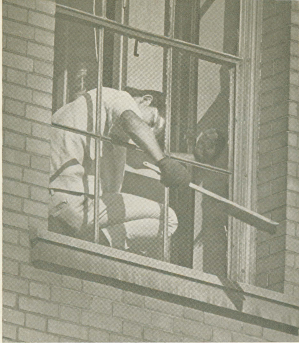
A building maintenance employee brushes broken glass from a window well at S.M.I. before plywood is installed. Note that four of the windows shown were broken by the concussion. (Photos by Dennis Connor and Gary Schulz.)
