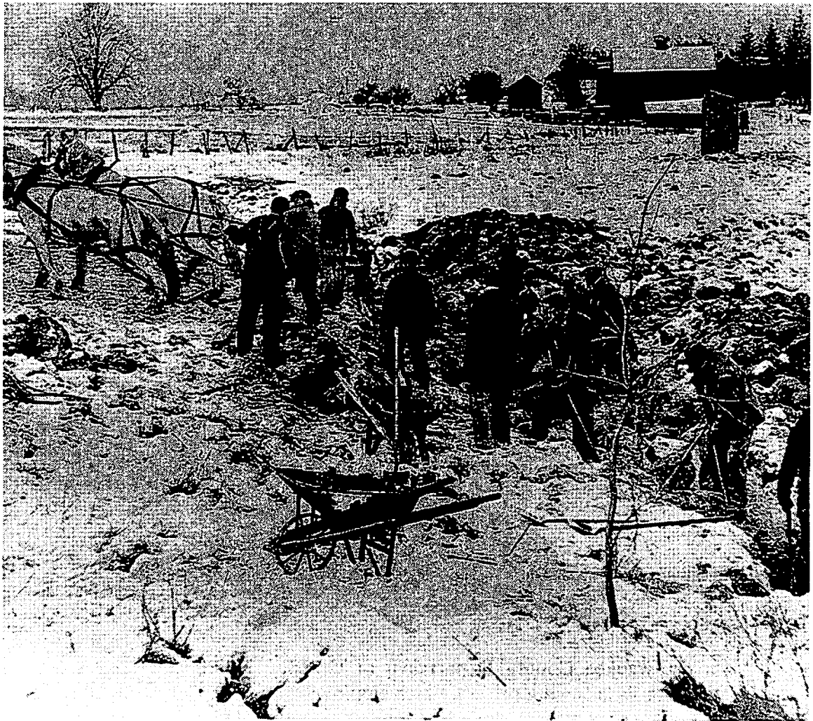
WPA workers clear land for the Village of Greendale using horses, wheelbarrows, and shovels.
