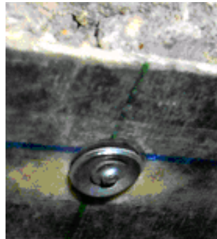
Figure 4.28. Over-driven fastener in the FRP strip
