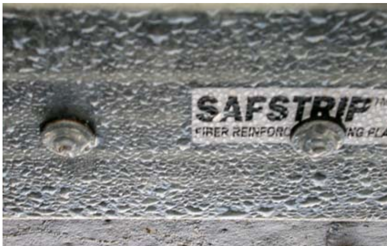
Figure 6.37. FRP strips covered with moisture (spring, 2003)
