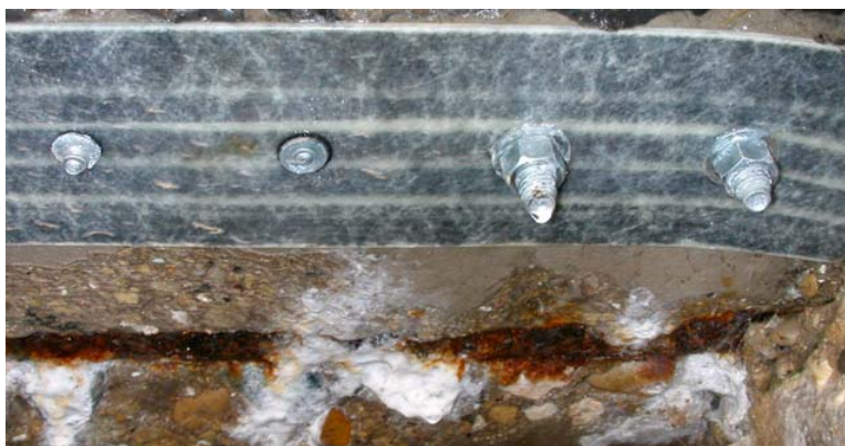
Figure 6.40. Original damaged area near the northern abutment
