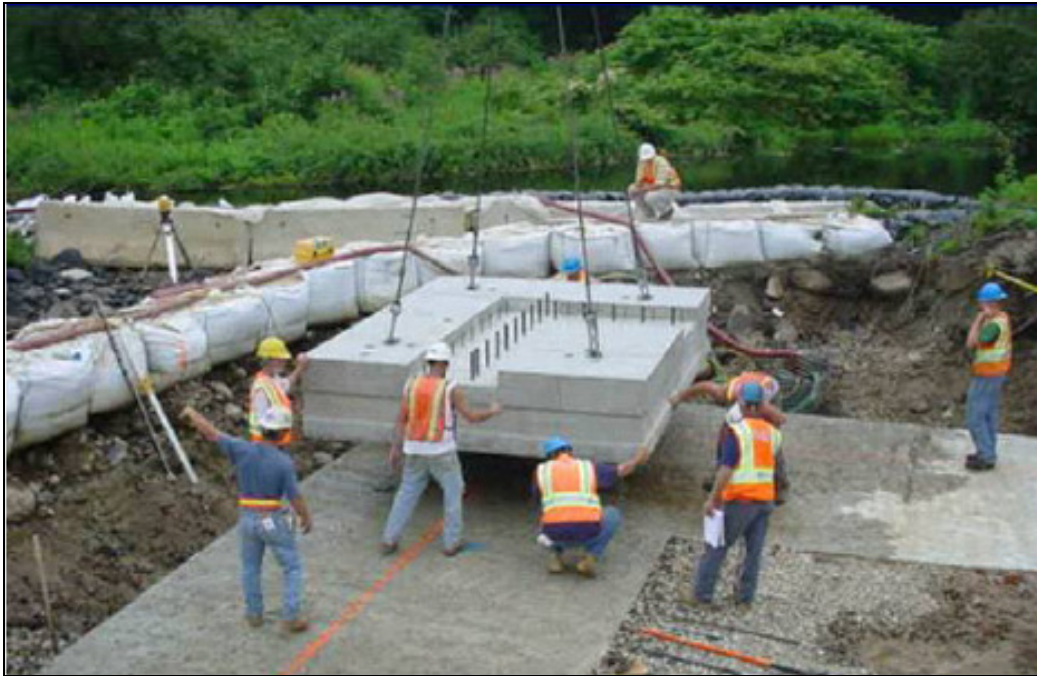
Figure 2-1 – Precast footing module with a shear key and splice detail getting placed on subfooting 4
