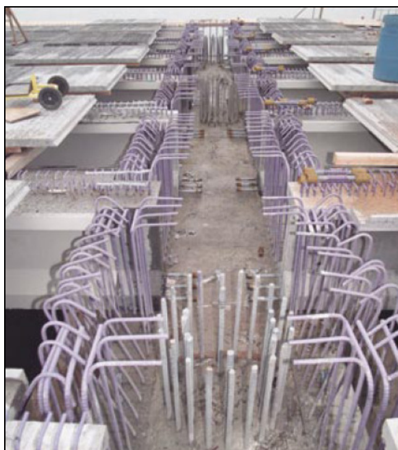
Figure 2-16 – Precast concrete cap shell shown with pile reinforcement and the girders in place, ready for concrete casting in the center region 28
