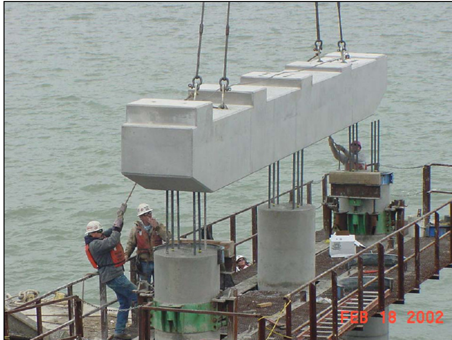
Figure 2-18 – Dowels protruding from the columns are inserted in the ducts in the cap 30
