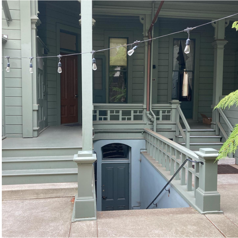
Figure 1.16. Image showing the basement entrance at the back of the Haas-Lilienthal House. The Haas-Lilienthal House Collection. Courtesy of San Francisco Heritage.
