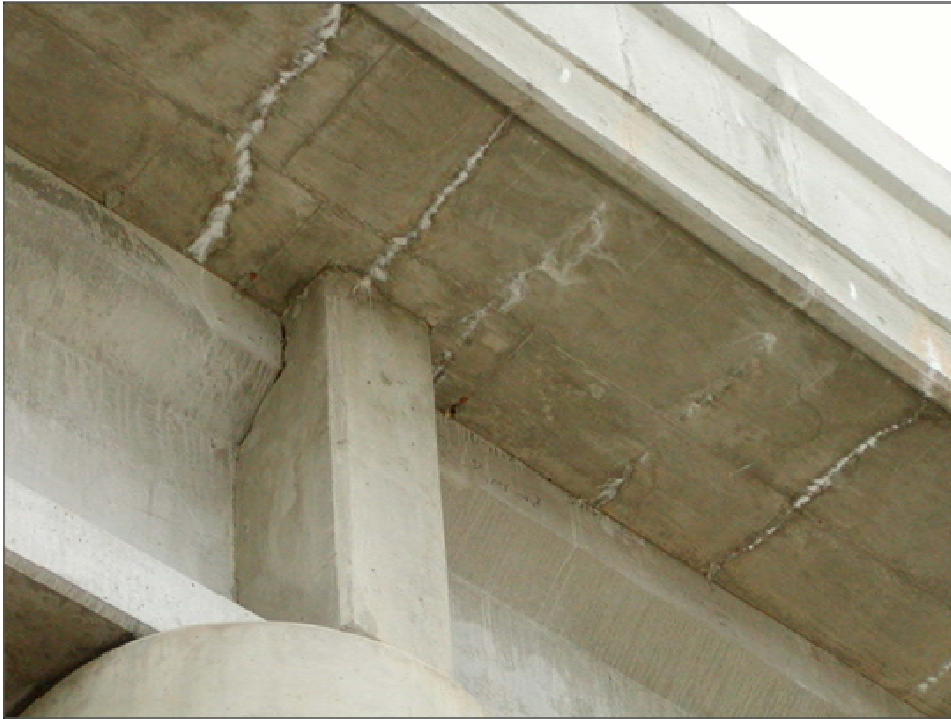
Figure 5.3 Cracking with Efflorescence (South Side of B-20-133 above Central Pier).
