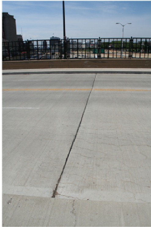
Figure 4.7 Bridge B-40-689: Longitudinal Cracks at the Construction Joint.
