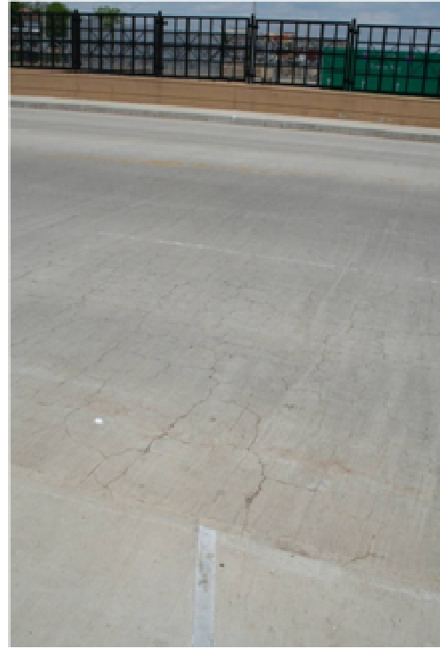
(b) B-40-686 Transverse Cracks
