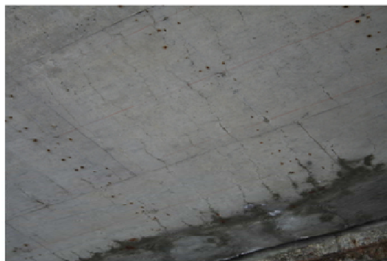
(b) B-67-293/294 Transverse Cracks
