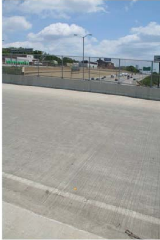
Figure 4.19 Bridge B-40-34 Deck Cracking (Transverse Cracks).
