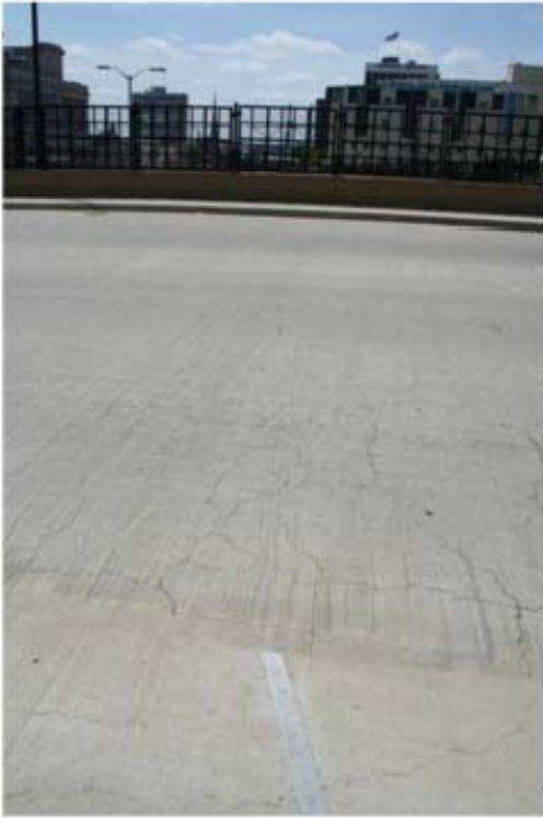
(a) B-40-686 Map Cracks
