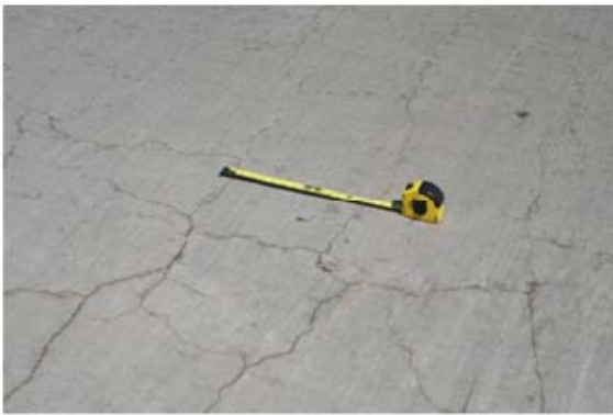
(c) B-40-692 Map Cracks
