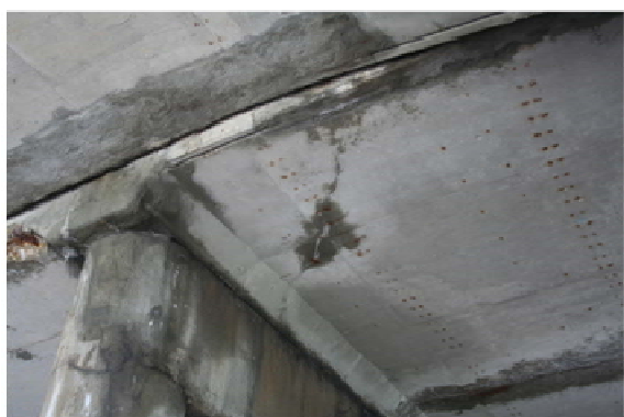
(c) B-67-293/294 Diagonal Cracks
