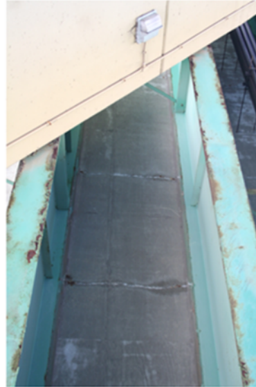
(b) B-40-429 Transverse Cracks on Bottom
