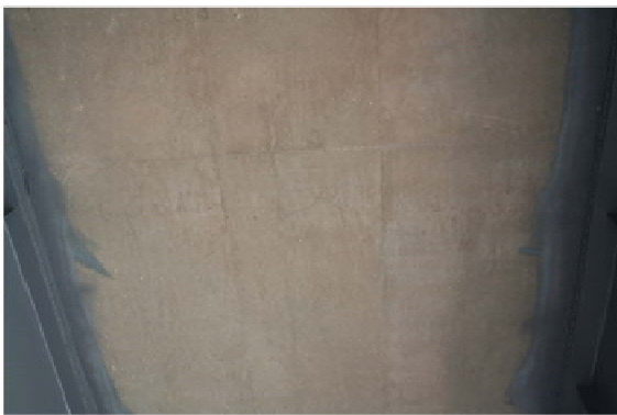
(c) B-67-134/135 Longitudinal Cracks
