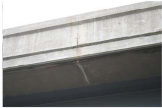
(b) B-67-134/135 Transverse Cracks at Barriers
