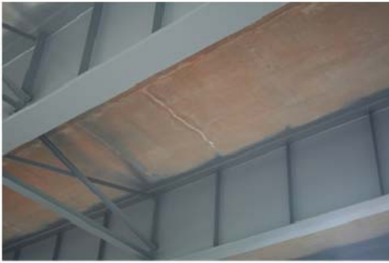
(a) B-67-134/135 Transverse Cracks
