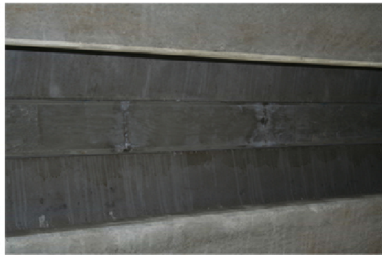
(b) B-67-296/297 Transverse Cracks
