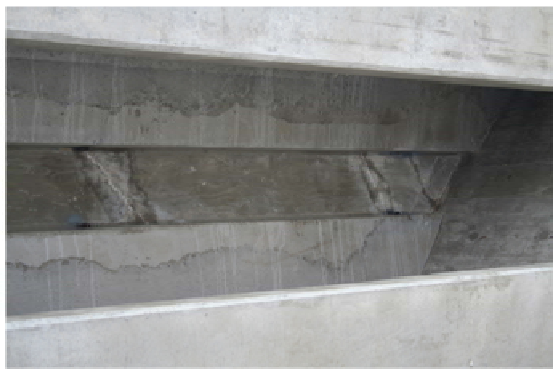
(c) B-67-296/297 Diagonal Cracks
