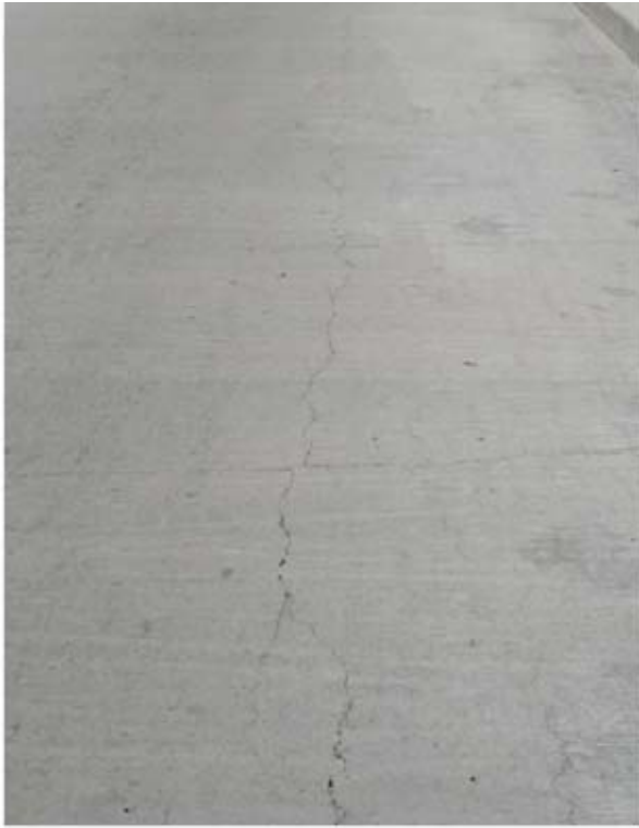
(a) B-40-692 Longitudinal Cracks
