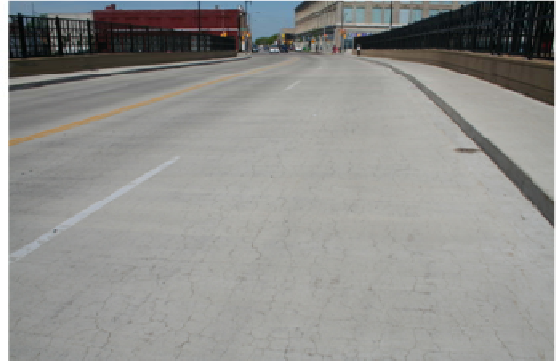
(b) B-40-689 Longitudinal Cracks
