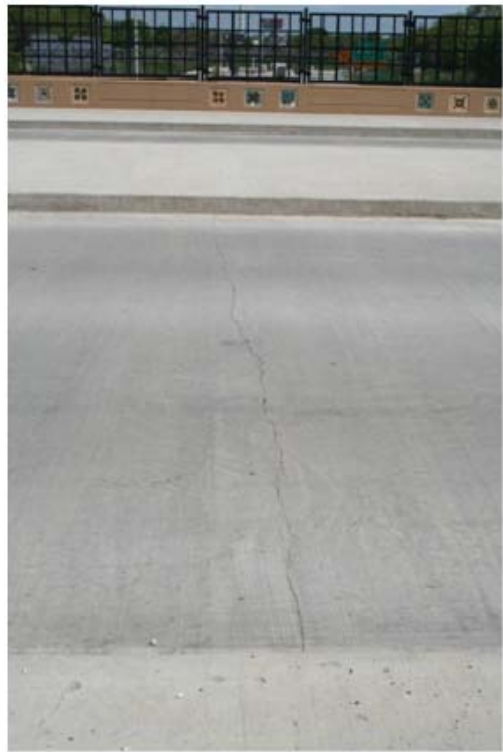
(b) B-40-692 Transverse Cracks
