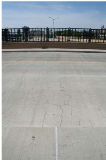
(c) B-40-689 Map Cracks
