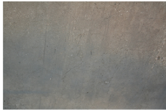
(c) B-67-134/135 Map Cracks
