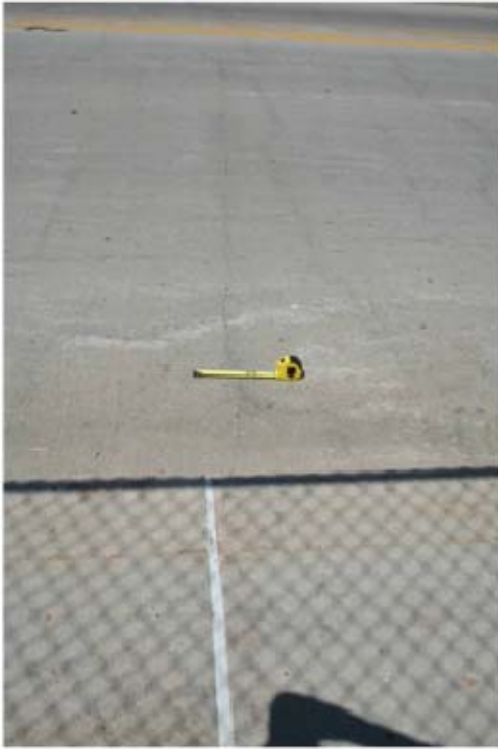
(a) B-40-429 Transverse Cracks on Top
