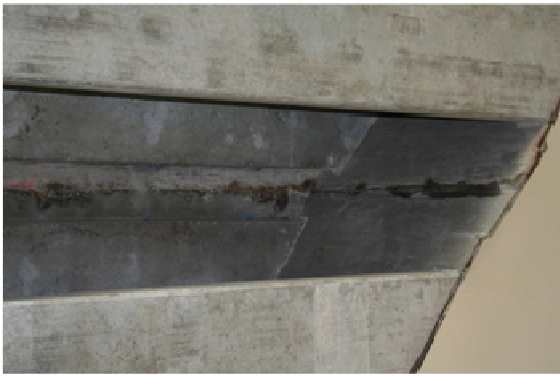
(a) B-67-296/297 Longitudinal Cracks
