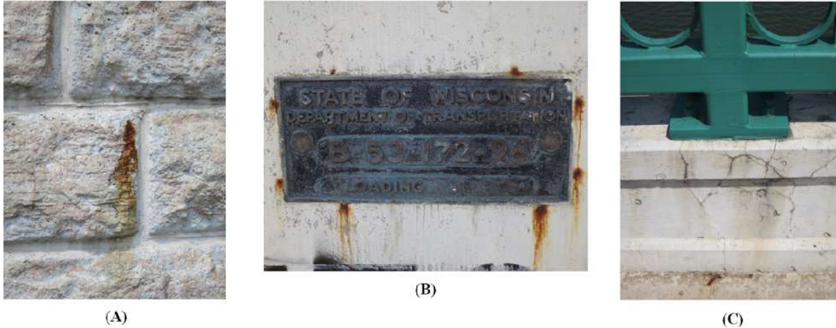
Figure 3-4: Examples of rust staining; (A) Exposed reinforcement on form lined surface, (B) Surrounding structural identification plaque, (C) Cracking near anchoring of steel guardrail.
