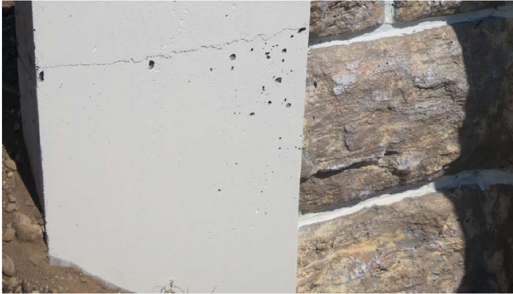
Figure 3-2: Discontinuities in coating film caused by surface voids.
