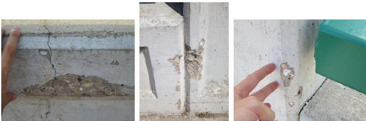
Figure 3-5: Examples of spalled concrete on the Portland Avenue Bridge (Beloit, WI).
