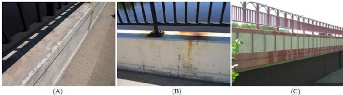
Figure 1-1: Examples of coating failures; (A) Peeling on Jefferson Bridge parapets, (B) rust bleeding/staining on Sauk City Bridge parapet, and (C) Color fading on Baraboo Bridge.
