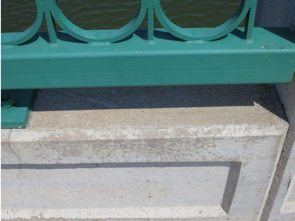
Figure 3-3: Loss of coating film on horizontal surface and the immediately adjacent vertical surface of a parapet.
