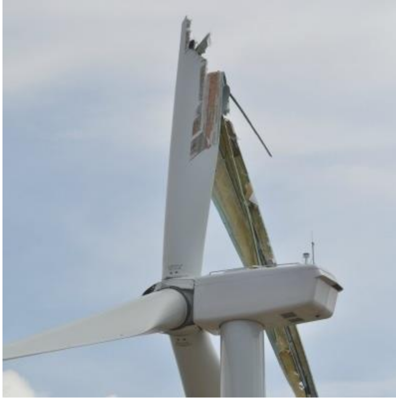
Figure 1: Photograph of a broken turbine blade at the Prairie Breeze wind farm in Nebraska [7].
