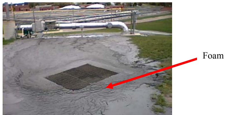
Figure 4: Acid Digester Foaming out the Top of the Digester (Reusser 2009)
