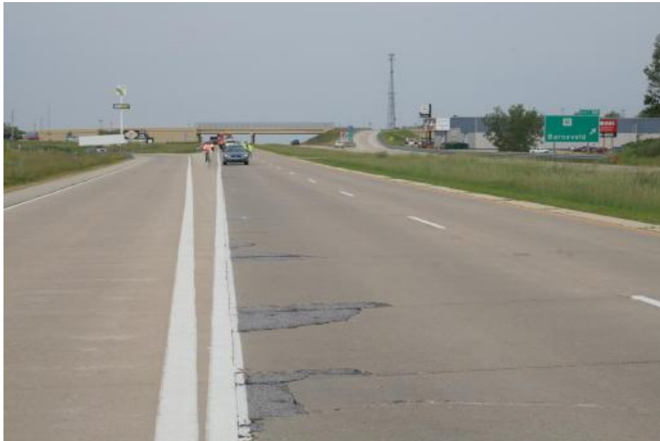
Figure 5.1 Patching in TIC Section Adjacent to New On-Ramp
