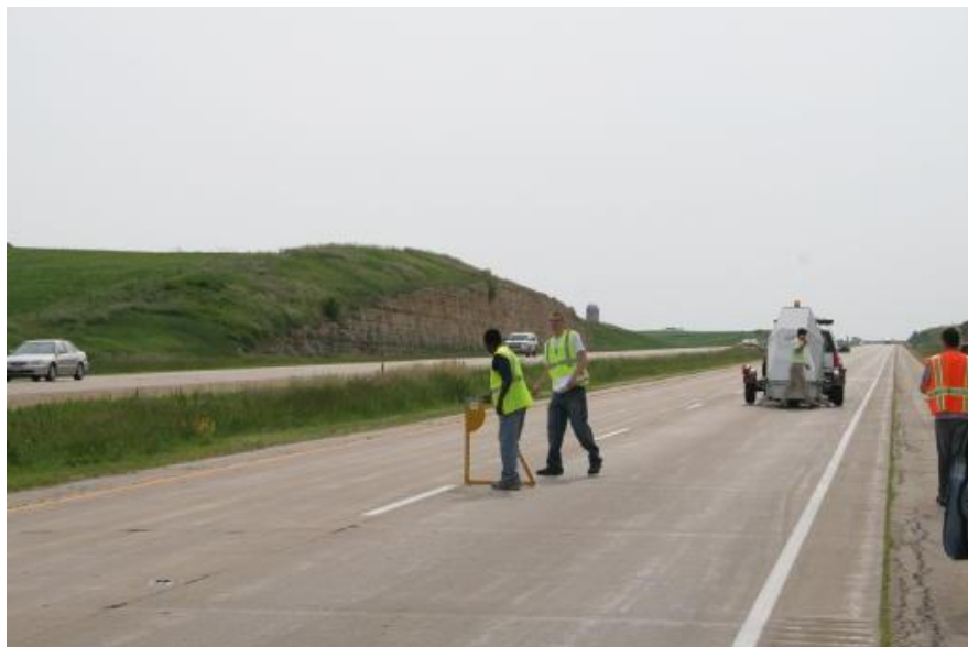
Figure 4.2 Longitudinal Fault Measurement on USH 18/151
