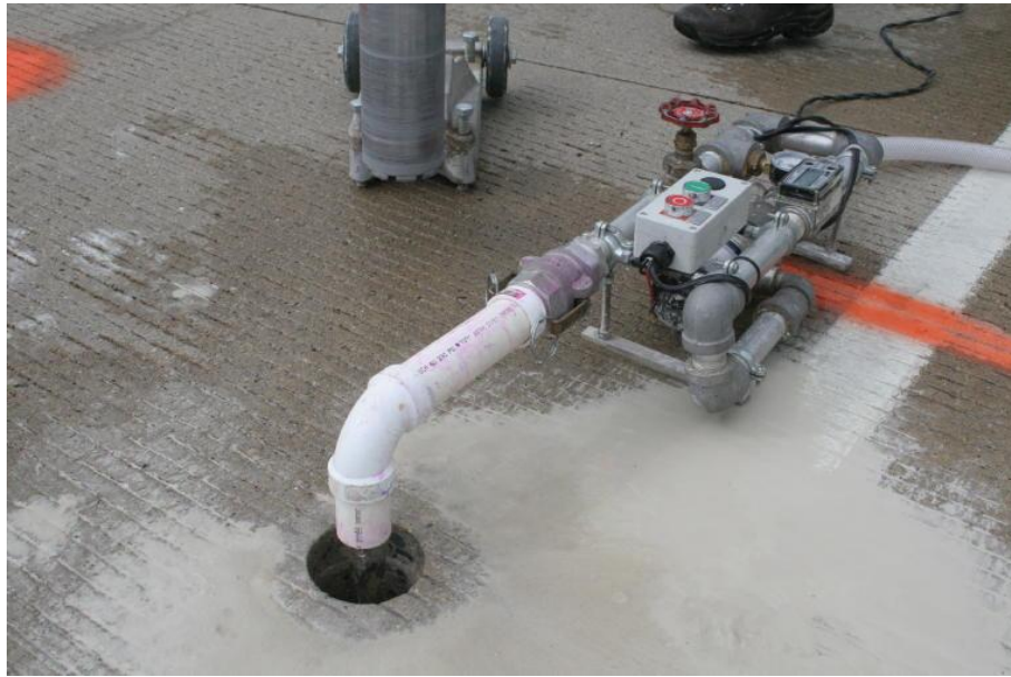
Figure 4.8 Water Flow Meter (USH 18/151)
