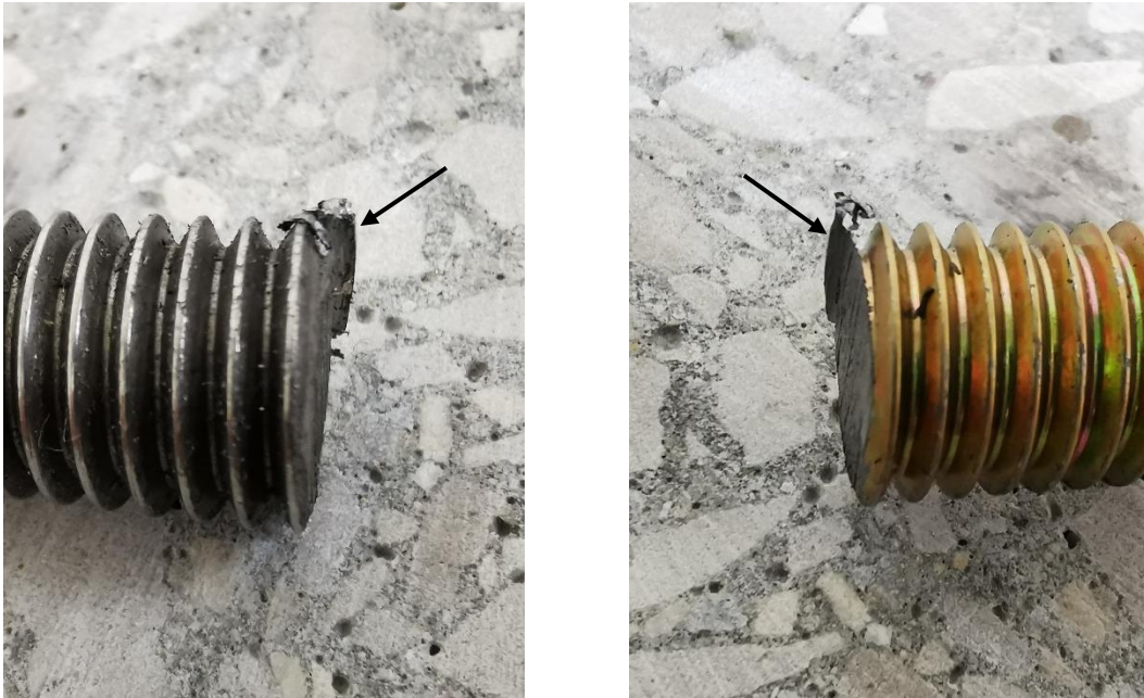
Figure V.1. Bent threads on an anchor rod.
