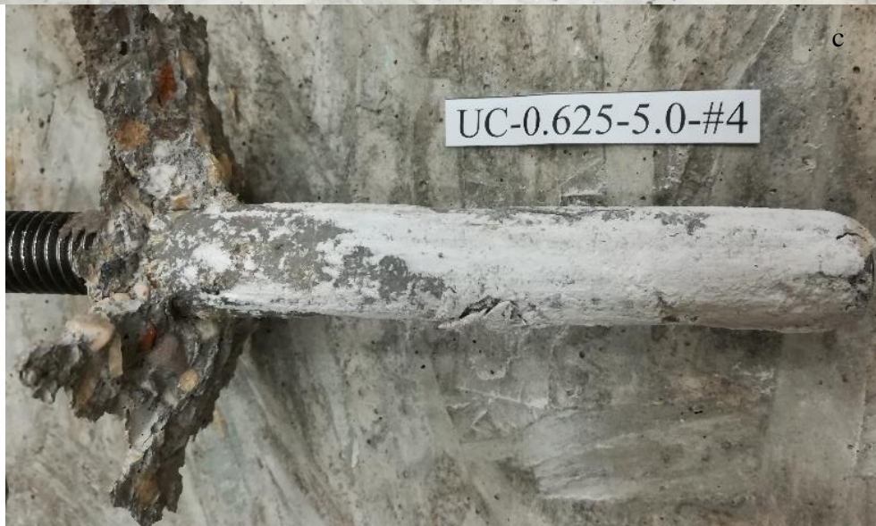
a) load-displacement behavior; b) cracked surface; c) partial cone bond failure. Figure VI.36. Observed behavior of Specimen UC-0.625-5.0-#4
