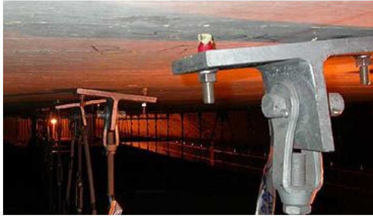
Figure 1.4. Adhesive anchors failure in a Boston Tunnel.
