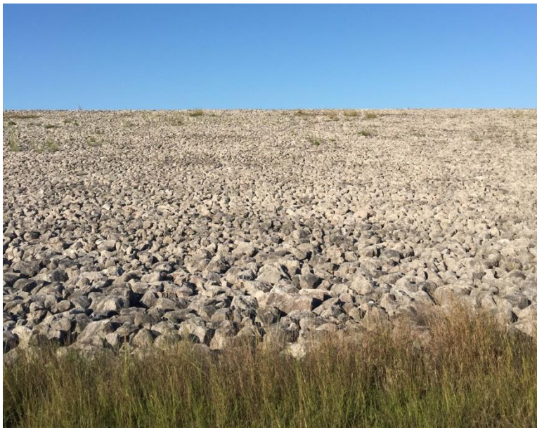
Figure A.4 The top figure shows the transition from the vegetative cell cover to the rock apron. The bottom image looks up the rock armored slope.
