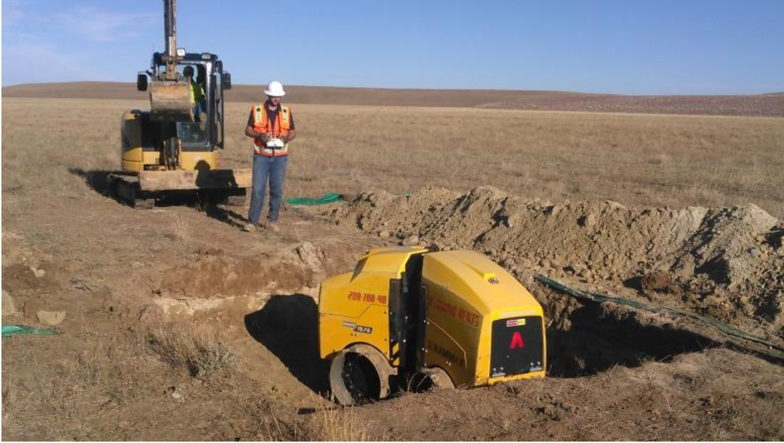
Figure B93 – Reconstruction of the Rn barrier and protective layers using a remote controlled sheep's foot compactor.
