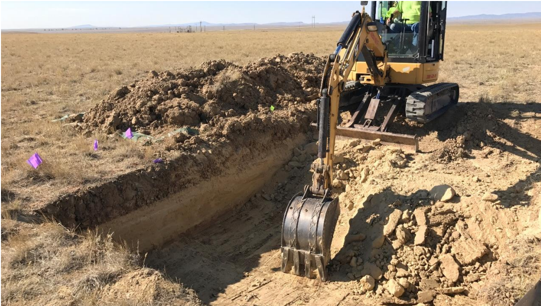
Figure B92 – Removal of the sandy overburden layer to expose the top surface of the Rn Barrier.
