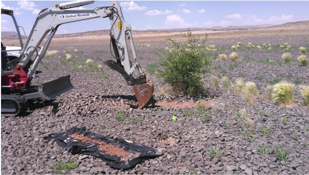
Figure 46 – Removal of the rip-rap layer to expose the top of the Rn barrier.
