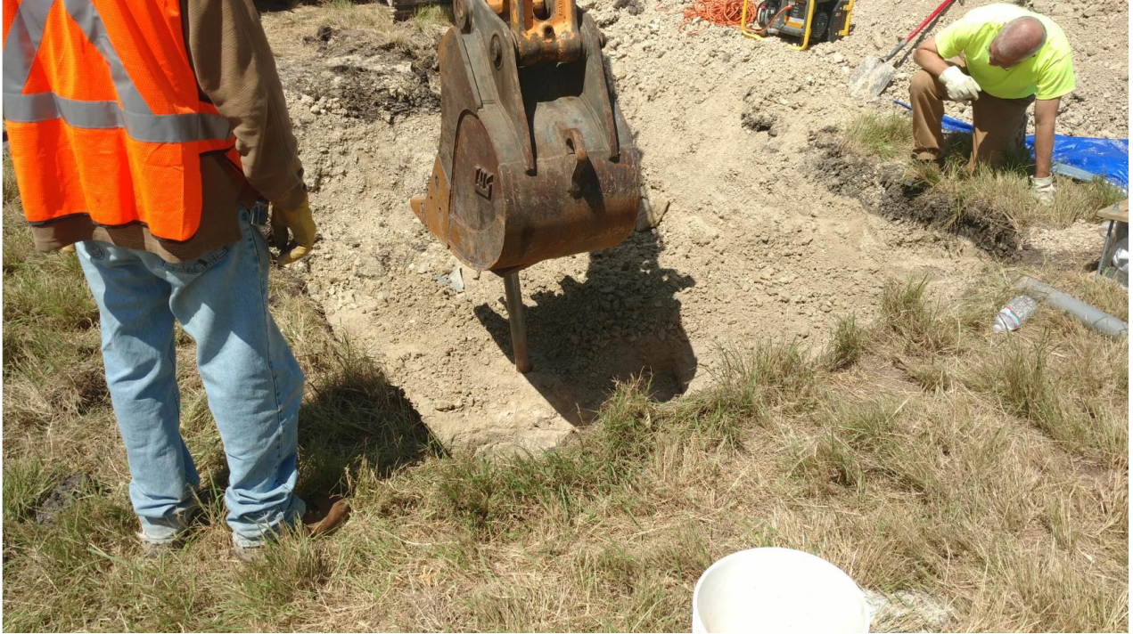
Figure 15 – Pushing a thin-walled tube sample through the Rn barrier with an excavator bucket.
