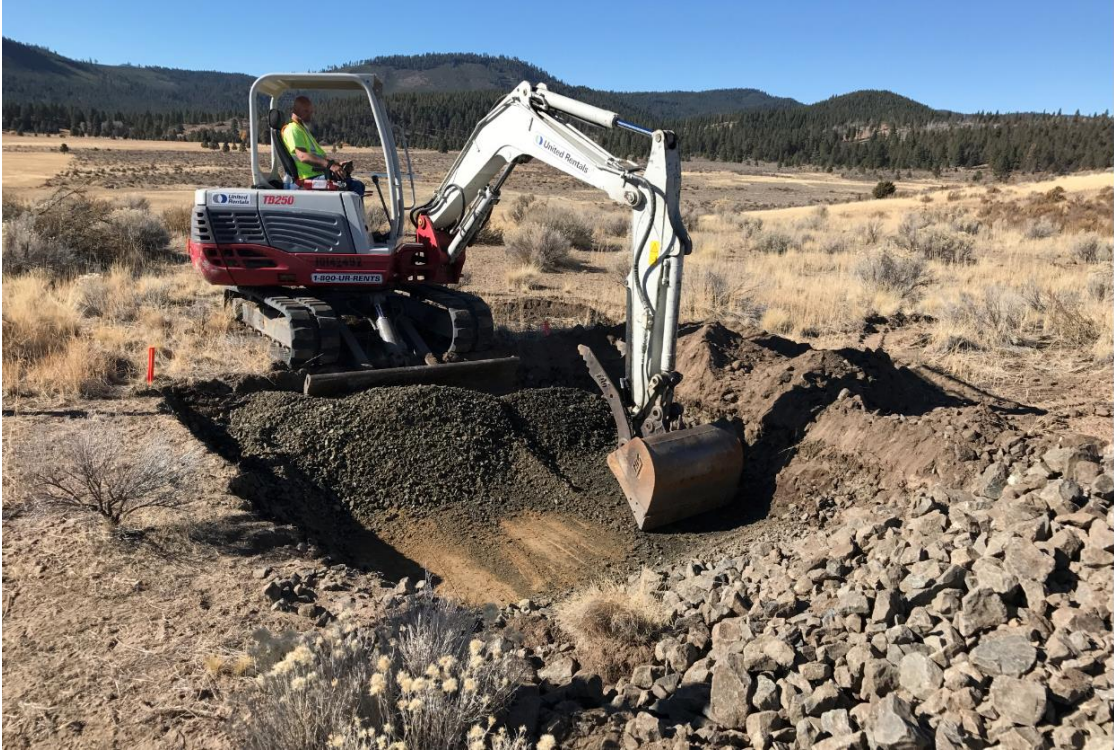
Figure 132 - Removal of the drainage layer to expose the top surface of the Rn Barrier.
