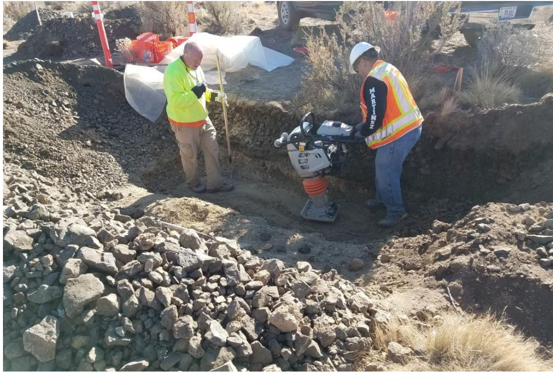
Figure 133 – Replacement and compaction of the Rn barrier soil using a hand operated compactor.
