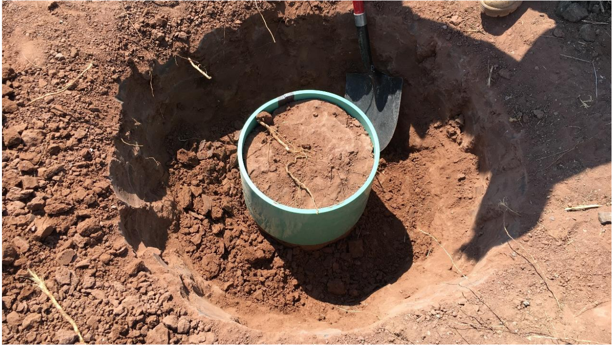
Figure 53 – Excavating a 350 mm diameter block sample from the Rn barrier with a shovel.
