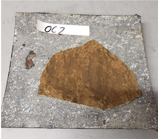
Figure A-42. Inside of a large ductile iron main obtained from Oak Creek. Minimal corrosion was observed on the exposed brown pipe wall.
