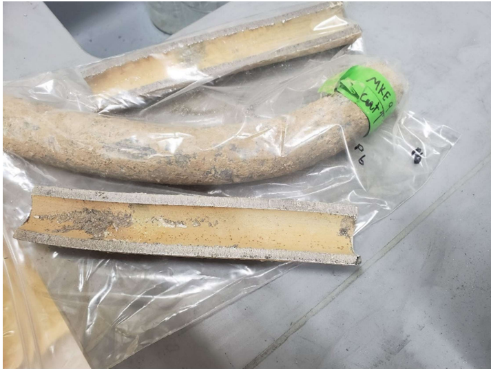
Figure A-19. Longitudinal cross-section of a lead pipe in Milwaukee (MKE-9-Pb). The pipe featured a goose-neck joint to attach to a copper pipe (MKE-9-Cu).
