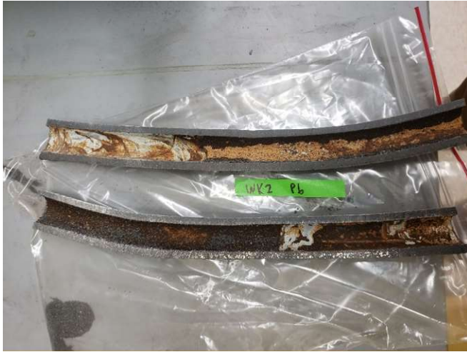
Figure A-52. Cross-section of a lead-lateral obtained from Waukesha displaying corrosion discoloration.
