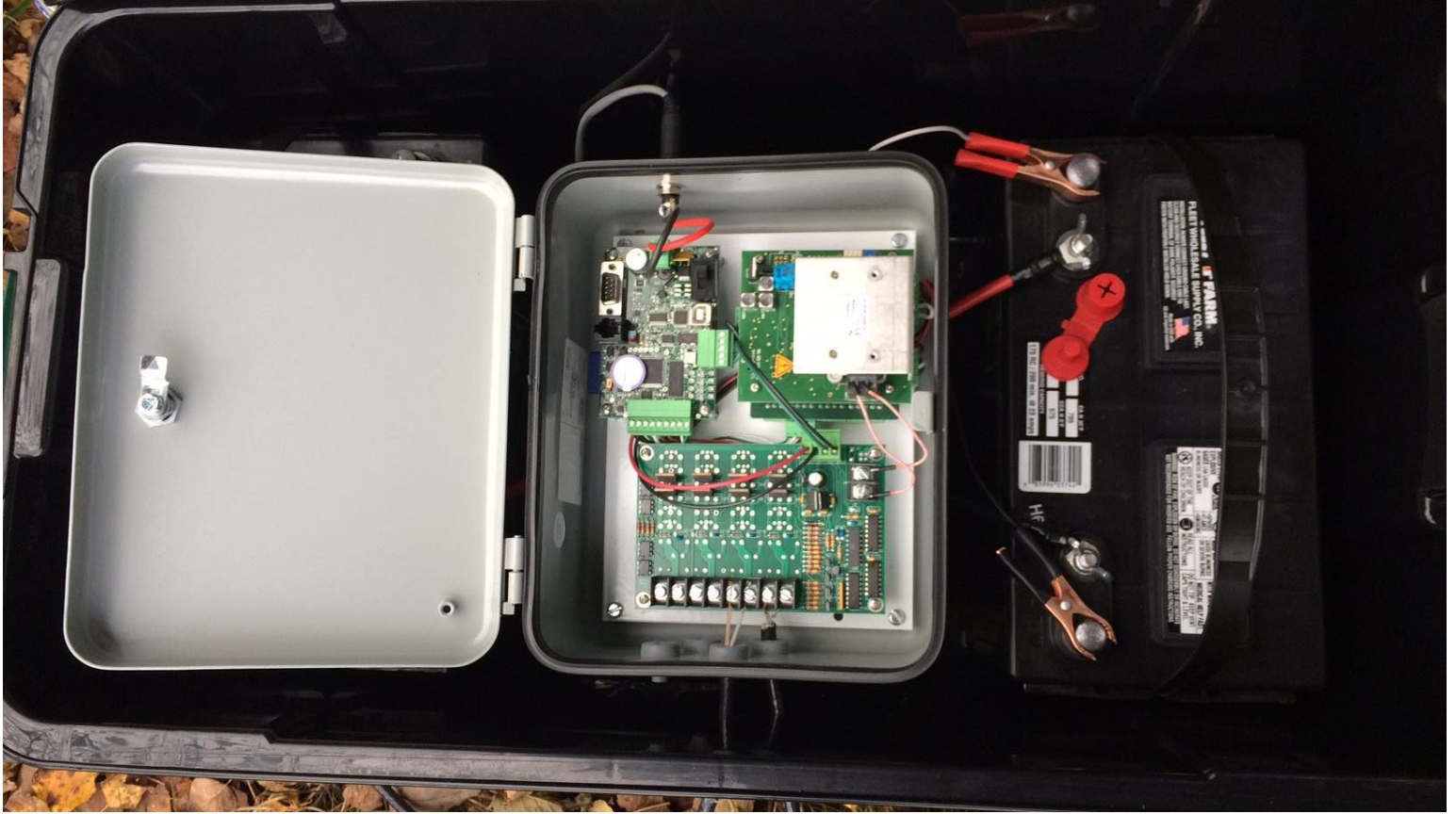
Figure 13. Oregon RFID® multi-antenna HDX reader box powered by two 12-volt deep cycle marine batteries connected in parallel.
