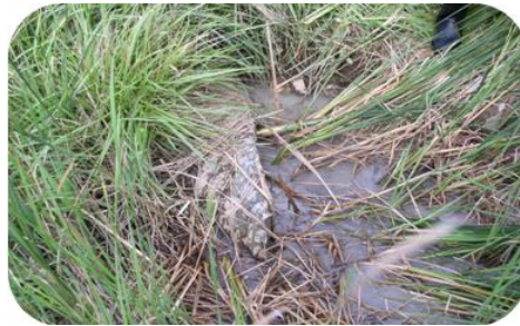
Figure 9.10: Total Failure of the Culvert End
