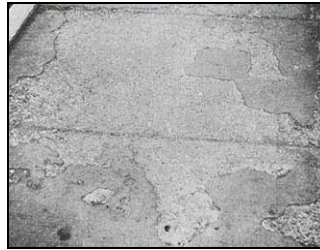
Figure 2.18: Scaling exposed on Concrete Surface. (Source: Photomac Construction industries, 2008)
