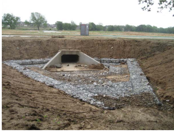
Figure 2.11: Riprap Basin to Protect Streambed and Stream Slope
