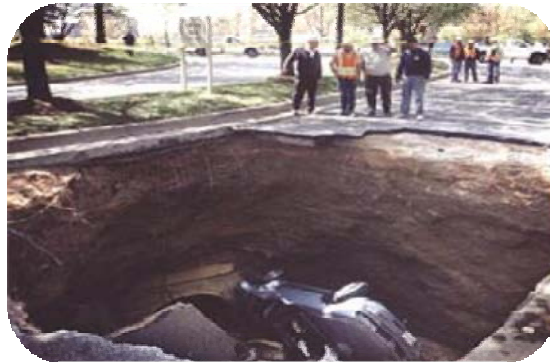
Figure 1.3: 84" Diameter CMP Failure in Maryland
