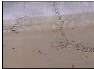
Figure 2.22: Honeycombing on a concrete surface. (Source: Department of Architectural Engineering, 2006)
