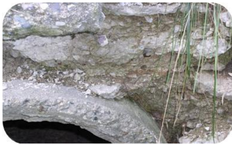
Figure 9.4: Failure of the Headwall due to Heavy Spalling
