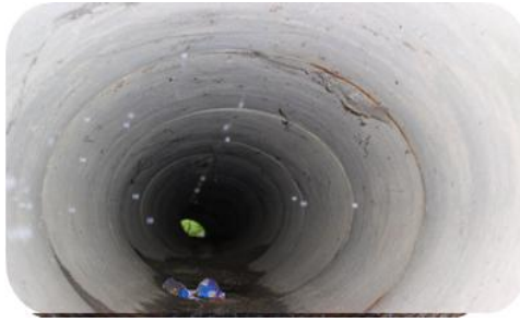
Figure 9.3: Misalignment of the Culvert
