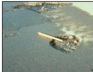
Figure 2.20: Spalling on a Concrete Surface. (Source: Caltrans, 2003)
