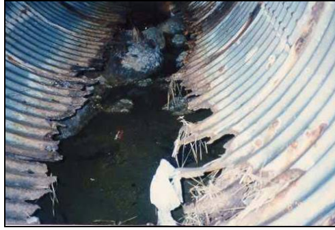
Figure 2.14: Deterioration due to Abrasion (Caltrans, 2003)
