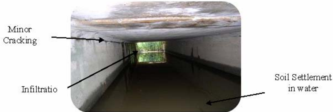
Figure 9.8: Condition of Culvert 31000131B04
