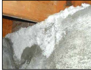
Figure 2.21: Formation of Efflorescence on a Concrete Surface. (Source: House Check, 2007)
