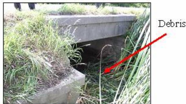
Figure 2.13: Debris at the Opening of the Culvert
