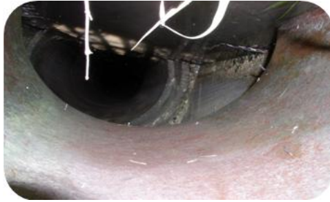
Figure 9.5: Significant Misalignment of the Culvert Structure
