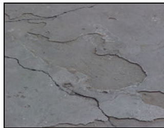
Figure 2.19: Delamination on a Concrete Surface. (Source: Concrete Restoration and Construction, 2007)
