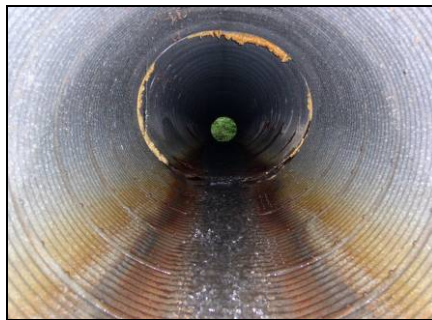
Figure 2.12: Corrosion in Culverts
