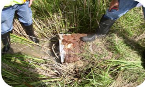
Figure 9.9: Corrosion on the Outside Surface of the CMP
