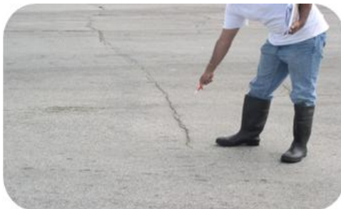
Figure 9.7: Cracks on the Roadway Surface
