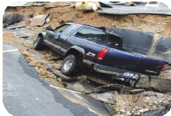
Figure 1.7: Failure of a 30-Year Old, 96" CMP in West Bountiful, Utah
