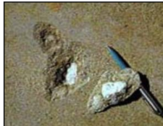
Figure 2.23: Pop-outs in a Concrete Structure. (Source: Concrete Sealers, Specialty Coatings and Consulting, 2006)
