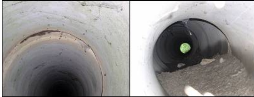
Figure 2.15: Culvert Pipe showing Cracks and Joint Separation
