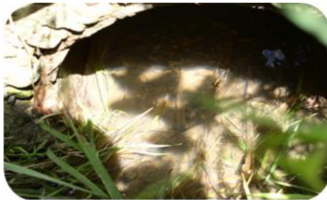
Figure 9.6: Vegetation and Heavy Spalling in the Headwall
