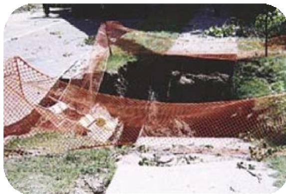
Figure 1.2: Culvert Failure in Muskegon, Michigan
