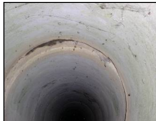
Figure 2.17: Transverse Cracks in a Culvert Pipe
