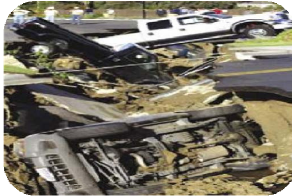
Figure 1.6: Failure of 30-Year Old CMP in Bakersfield, California
